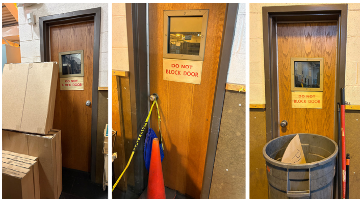
Figure 3. Blocked Inspection Service Doors
