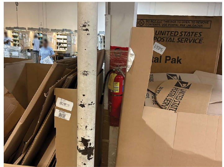
Figure 6. Blocked Fire Extinguisher
