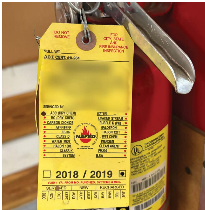
Figure 5. Fire Extinguisher Missing Annual Inspection
