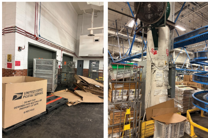
Figure 6. Blocked Elevators and Electrical Panel
