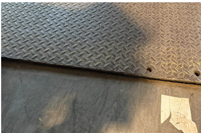
Figure 8. Steel Decking in Need of Re-bolting
