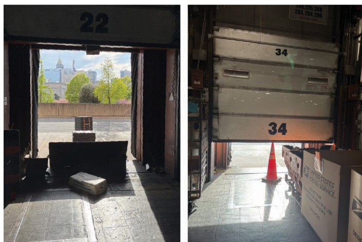
Figure 7. Inoperable Dock Plate and Door Opener
