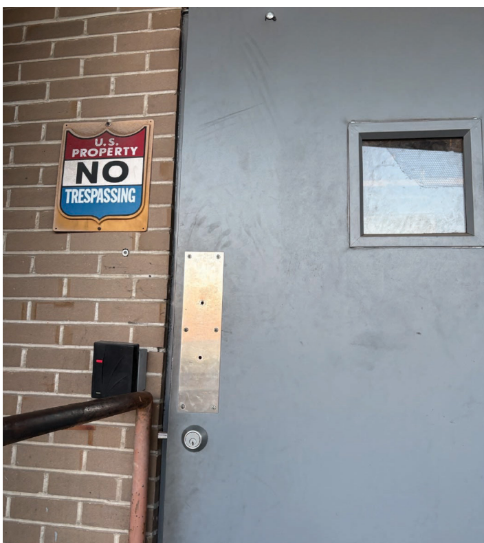
Figure 9. Employee Access Door Propped Open
