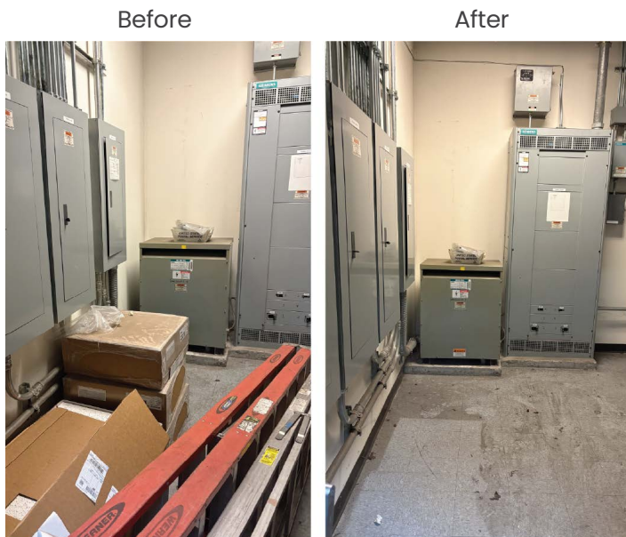
Figure 5. Blocked Electrical Panels
