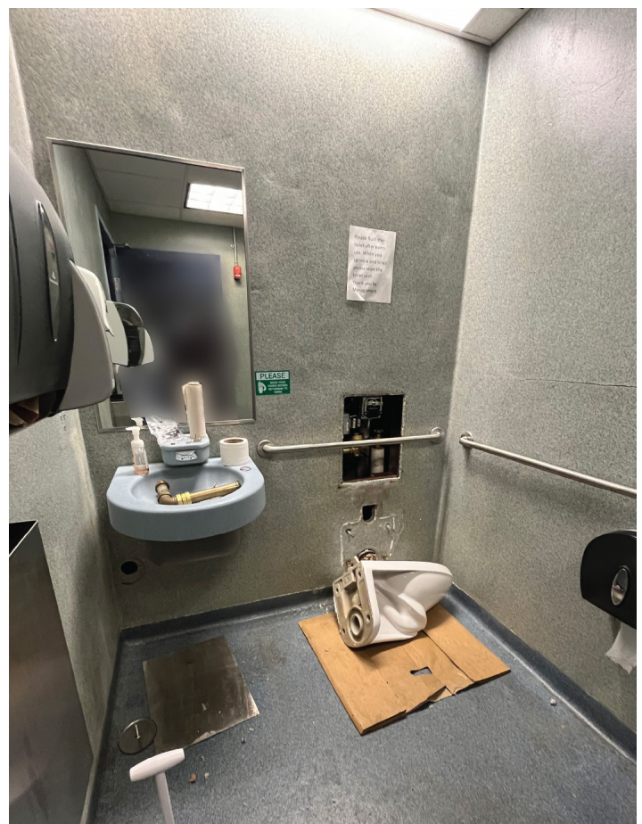
Figure 1. Plumbing Issues at Manhattan VMF
