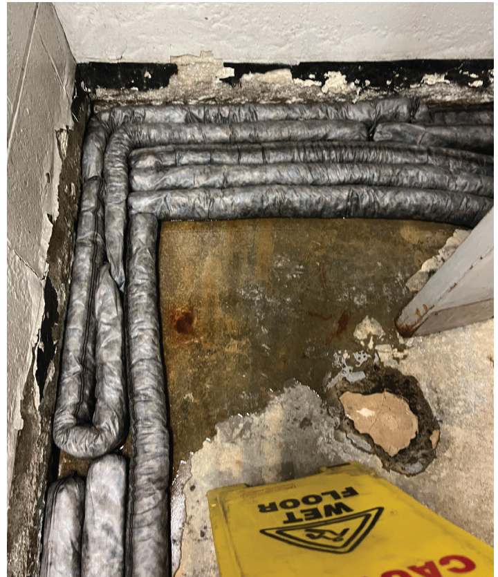
Figure 3. Unabated Leak With Absorbing Pads and Caution Sign Workarounds at Boston P&DC
