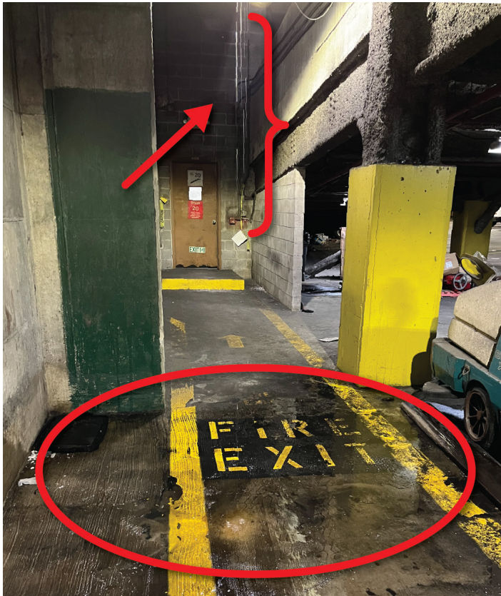
Figure 2. Water Leak in Basement at Morgan P&DC
