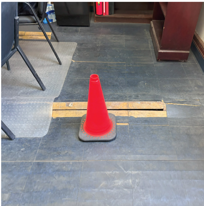
Figure 3. Damaged Floor in Manager's Office
