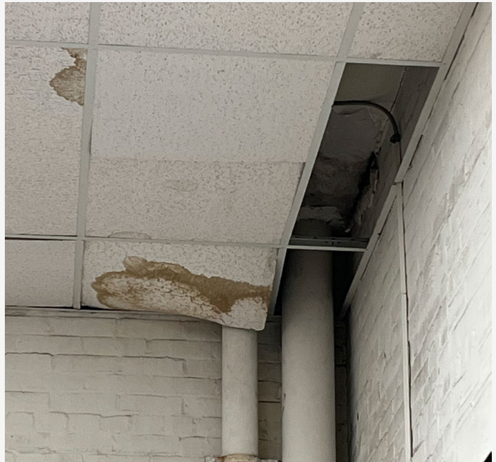
Figure 8. Stained, Missing, and Damaged Ceiling Tiles.
