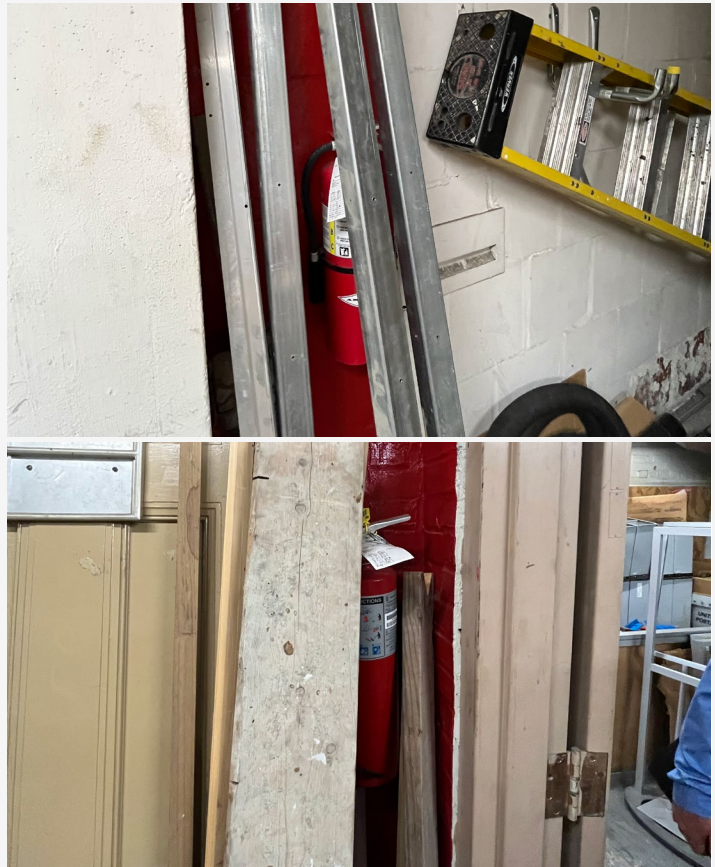
Figure 4. Blocked Fire Extinguishers.
