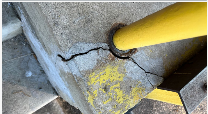
Figure 5. Damaged Concrete on the Loading Dock Platform.
