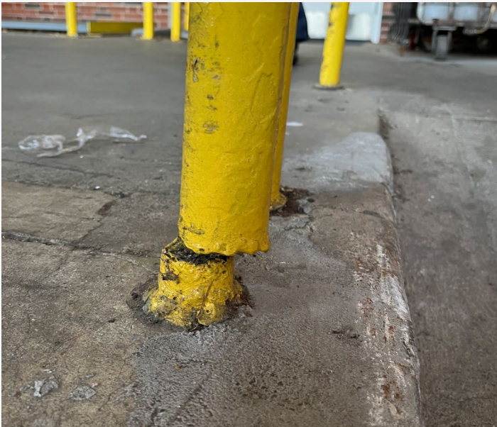
Figure 6. Broken Handrail Post on the Loading Dock Platform.
