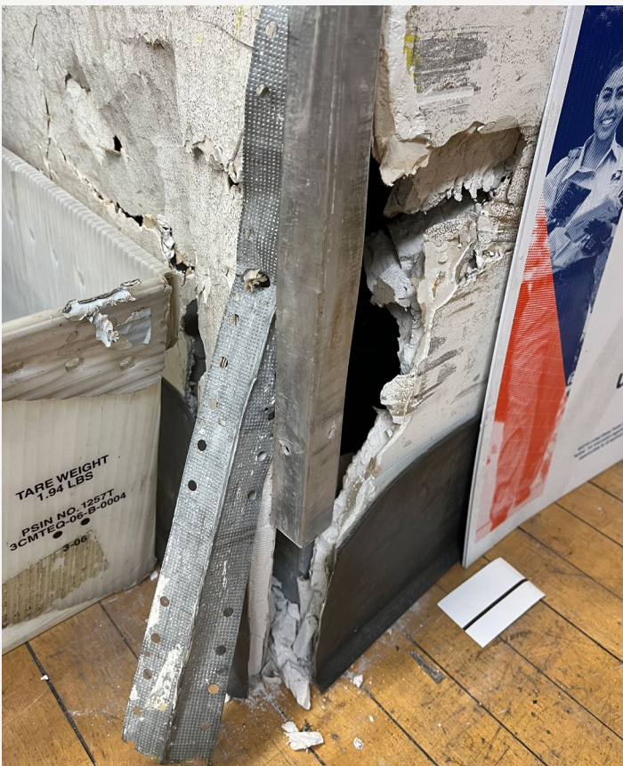
Figure 7. Drywall Damage in Workroom Area.
