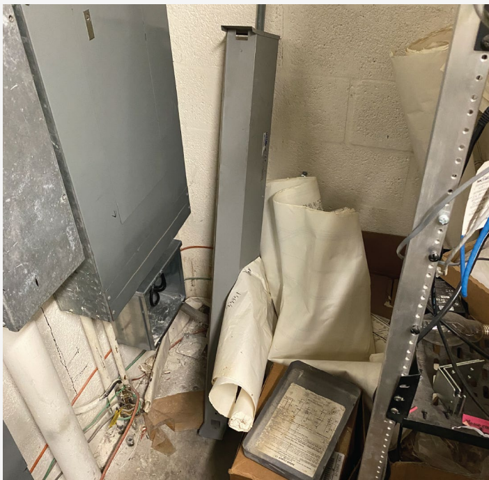
Figure 3. Blocked Electrical Panel
