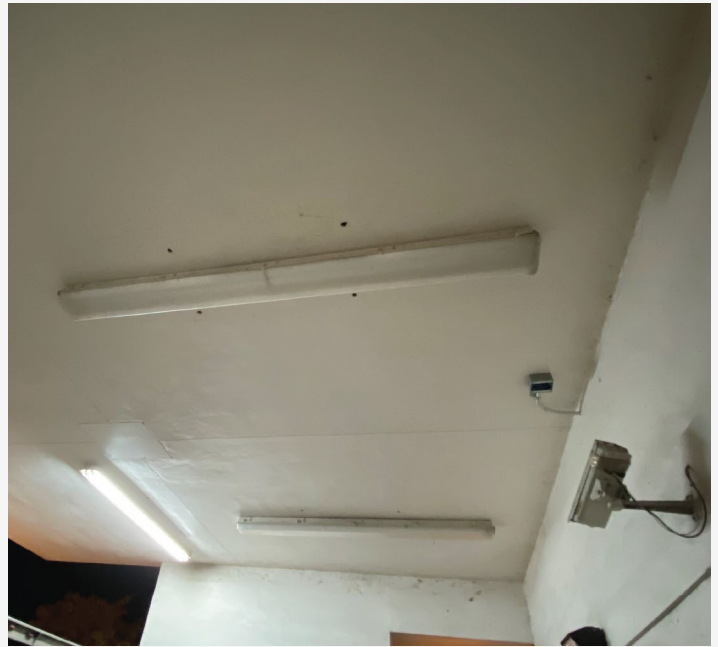
Figure 4. Non-working Dock Lights
