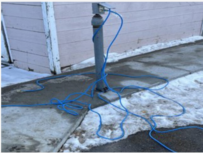
Figure 4. LLV Cords Scattered Across Sidewalk
