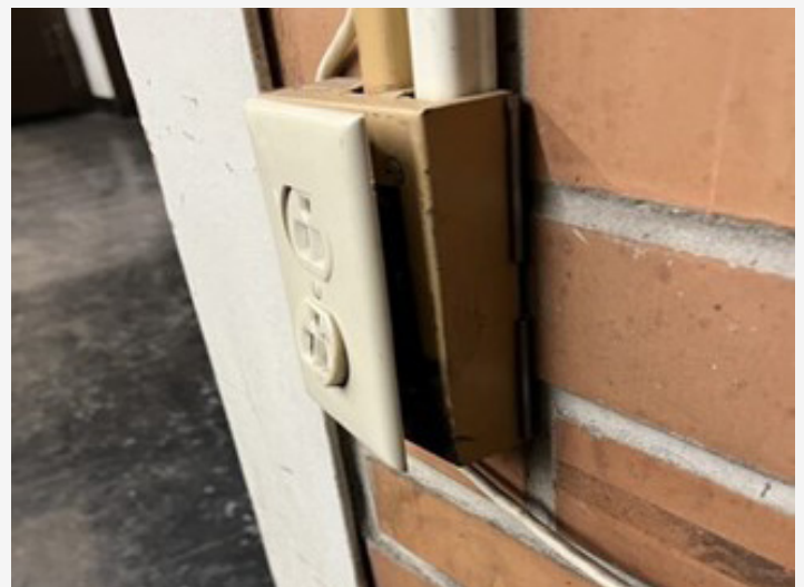
Figure 6. Broken Electrical Outlet
