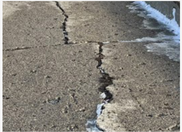
Figure 5. Uneven Sidewalk Creating Trip Hazard
