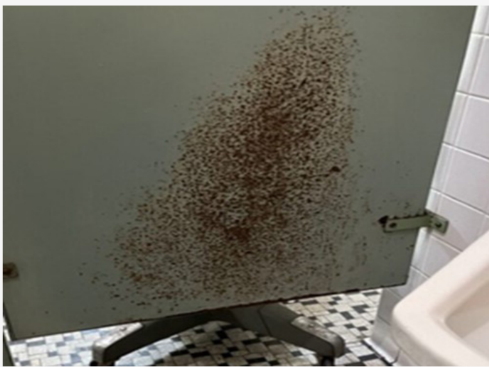
Figure 7. Panel Covered in Rust
