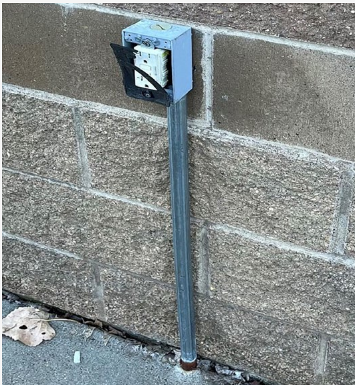
Figure 5. Example of a Damaged Electrical Outlet Cover
