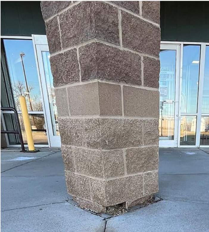
Figure 7. Damaged Column Base
