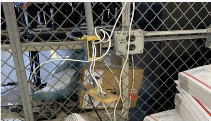
Figure 8. Exposed Wiring in the Registry Cage
