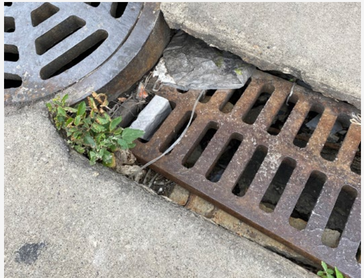
Figure 11. Misaligned Ground Plate in Parking Lot
