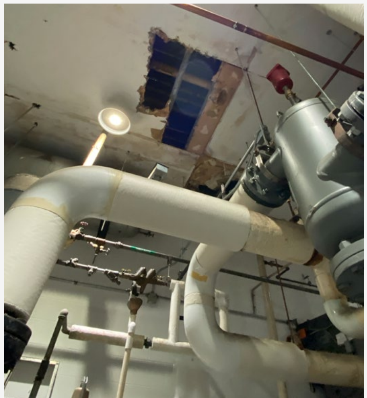
Figure 14. Roof Leak in Boiler Room
