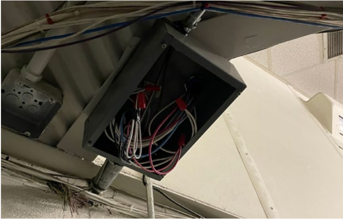
Figure 7. Exposed Wiring Near Equipment Room
