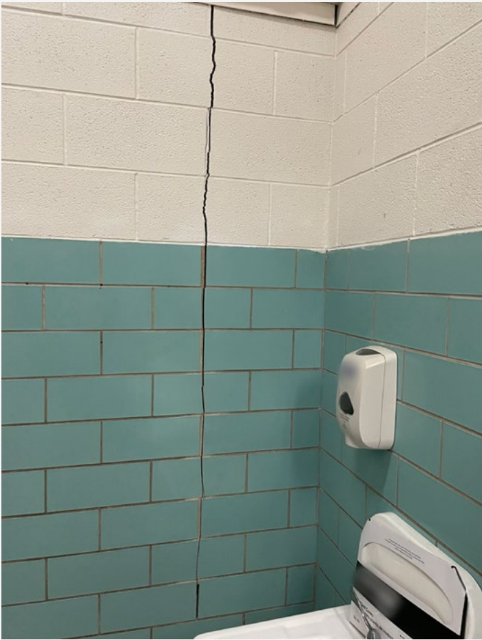
Figure 13. Crack on Wall in Men’s Restroom
