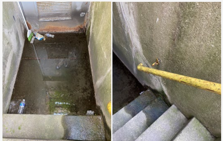
Figure 12. Standing Water and Damaged Handrail Outside Basement Door
