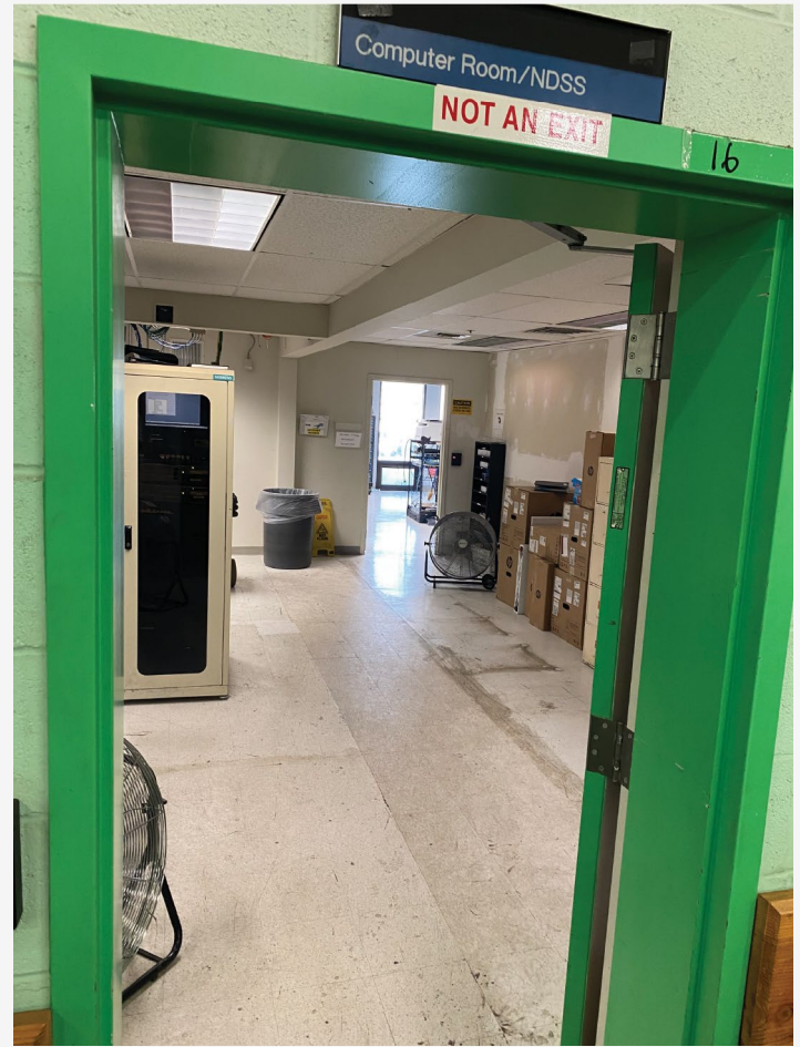
Figure 11. Unsecured Server Room Door
