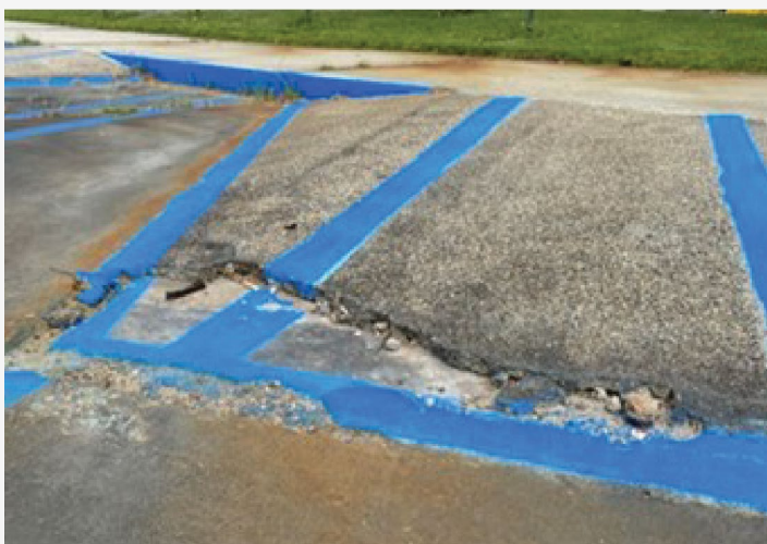
Figure 6. Handicap Ramp With Crumbling Asphalt
