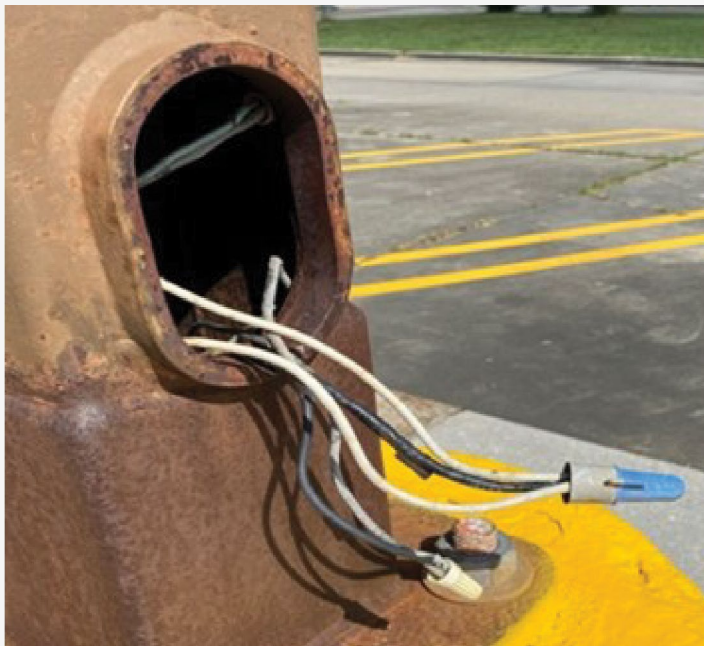
Figure 5. Light Pole in Customer Parking Lot With Exposed Wiring
