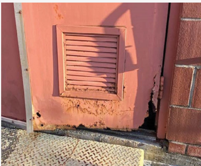
Figure 9. Rusted and Damaged Exterior Storage Room Door
