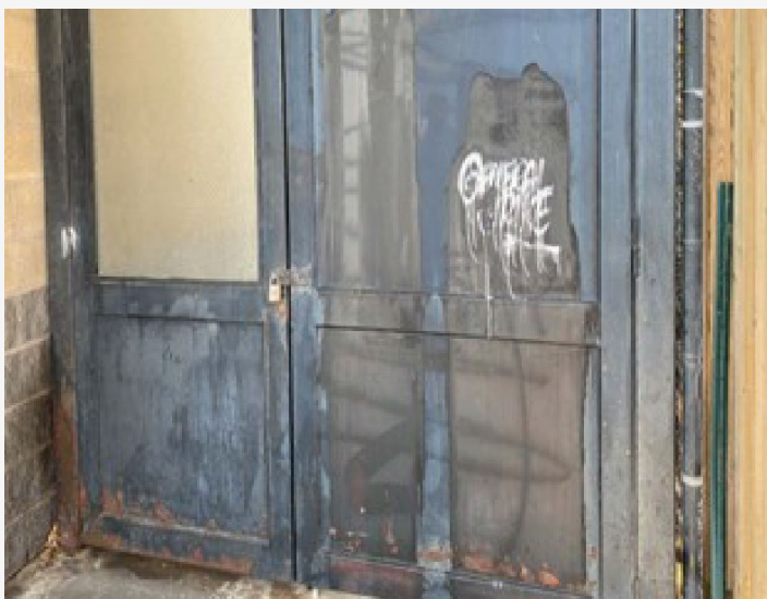
Figure 8. Graffiti on the Front, Retail Side of the Facility
