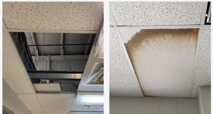
Figure 6. Examples of Missing and Stained Ceiling Tiles
