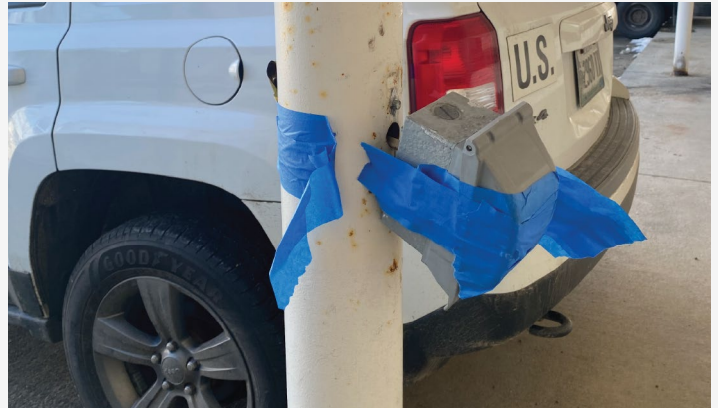
Figure 5. Broken and Unsecured Electrical Outlet
