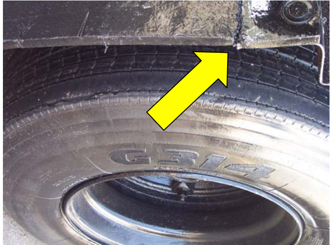
The broken frame on this leased trailer is an out of service deficiency. Photograph taken at the New Jersey International Bulk Mail Center May 1, 2002.
