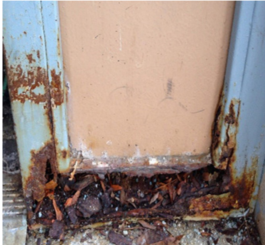
Figure 7: Deteriorating Door Frame
