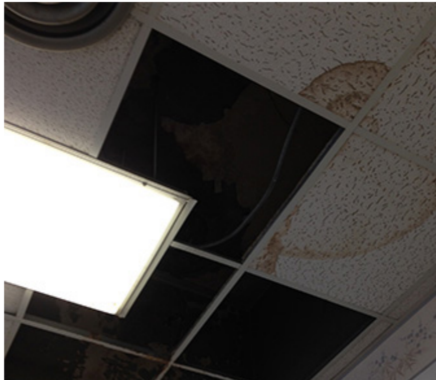
Figure 9: Missing Ceiling Tile
