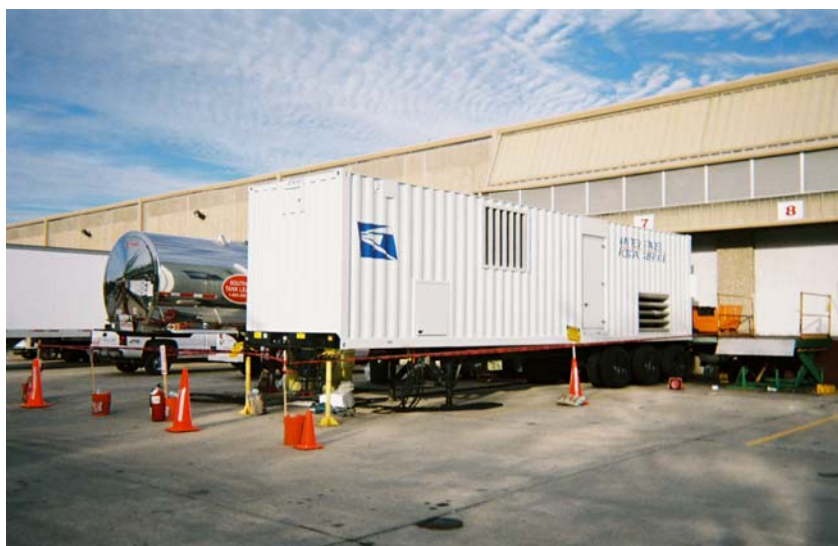
Photograph 3: Electrical Generator and Fuel Supply Tank in Use
