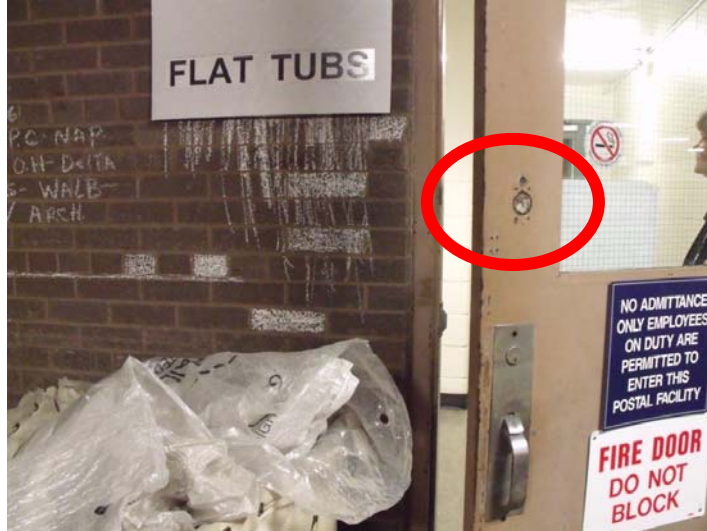
Illustration 4: Unsecured Door at the Toledo P&DC with Broken Lock. Photograph taken on 4/9/2010.
