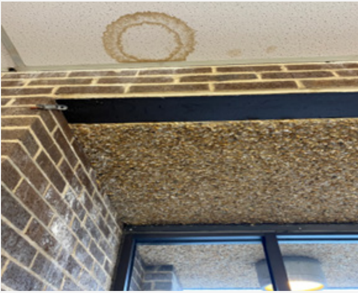
Figure 6. Stained Ceiling Tile and Dirty Wall in Lobby
