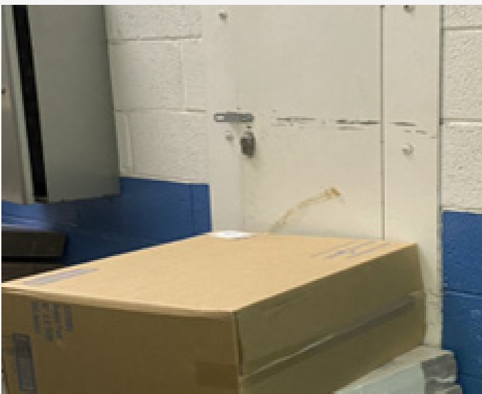
Figure 3. Blocked Electrical Panel
