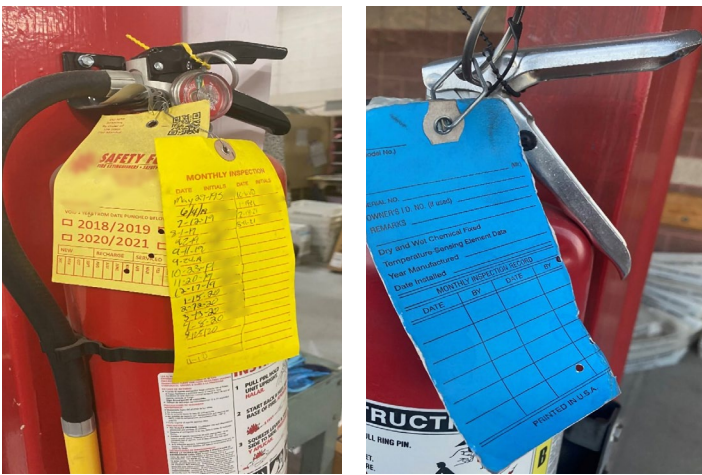
Figure 3. Fire Extinguishers Missing Annual or Monthly Inspections
