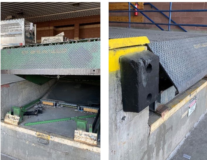
Figure 4. Broken Dock Lifts
