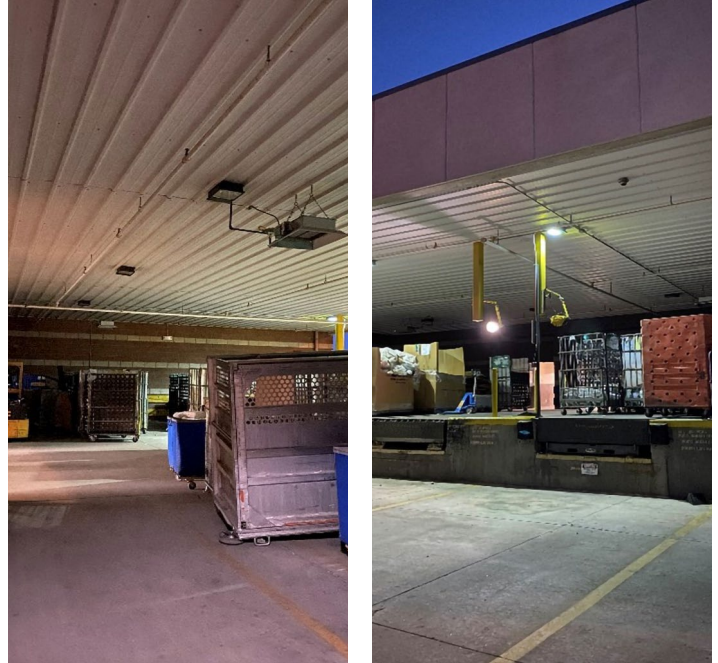
Figure 5. Non-Working Dock Lights
