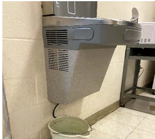
Figure 10. Water Fountain in Breakroom
