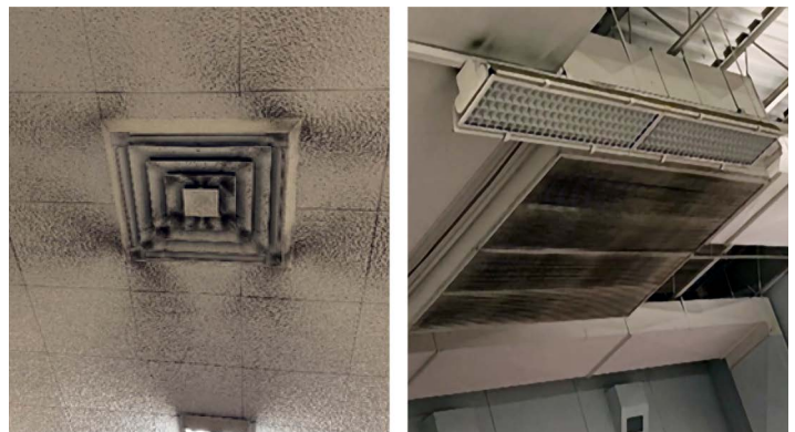
Figure 5. Dirty Air Vents
