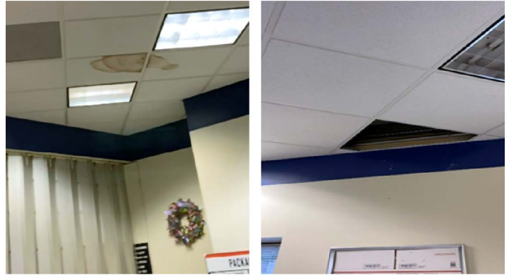
Figure 4. Damaged or Missing Ceiling Tiles
