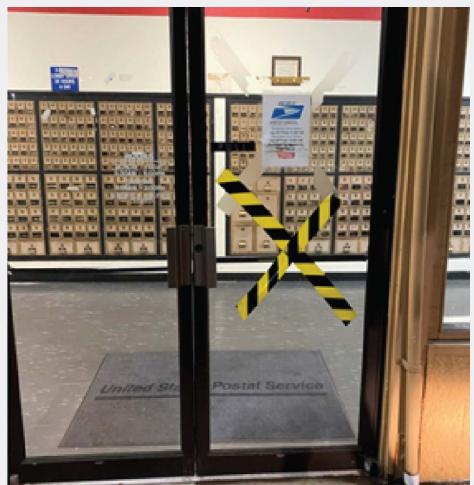
Figure 2. Non-Functioning Taped Lobby Door
