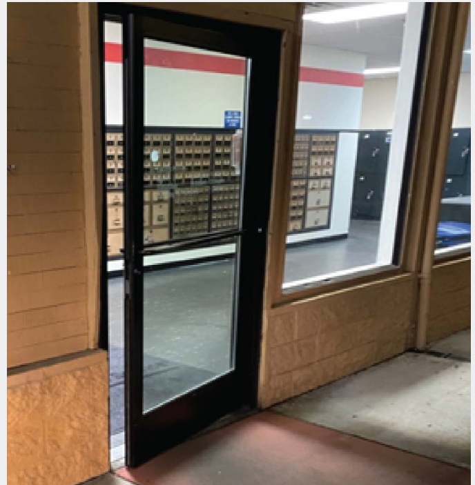
Figure 1. Door That Does Not Close Completely
