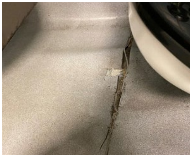
Figure 2. Cracked Flooring in Men's Restroom
