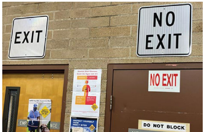
Figure 4. No Illuminated Exit Signs
