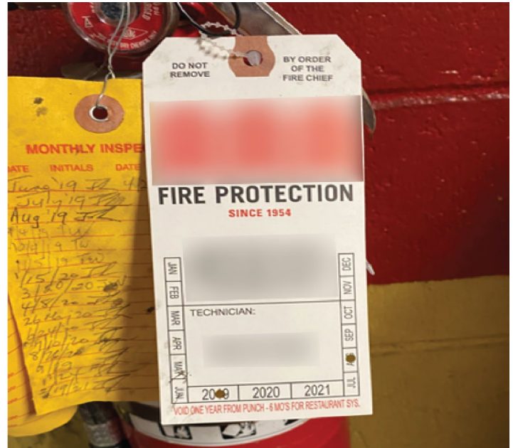
Figure 3. Portable Fire Extinguisher Missing Annual Inspections
