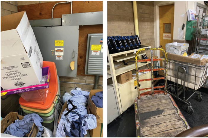
Figure 1. Blocked Electrical Panel and Inspection Service Door
