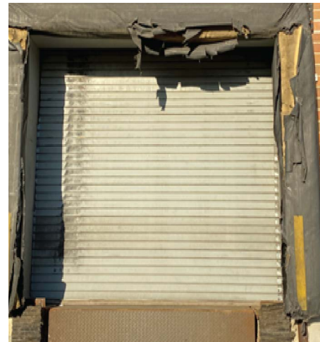
Figure 6. Padding Around Dock Door
