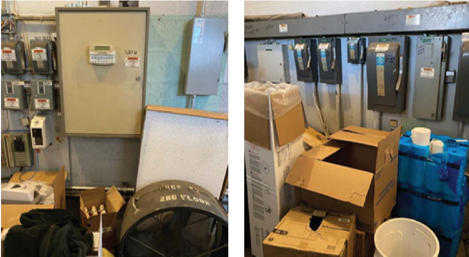
Figure 11. Blocked Electrical Panels
