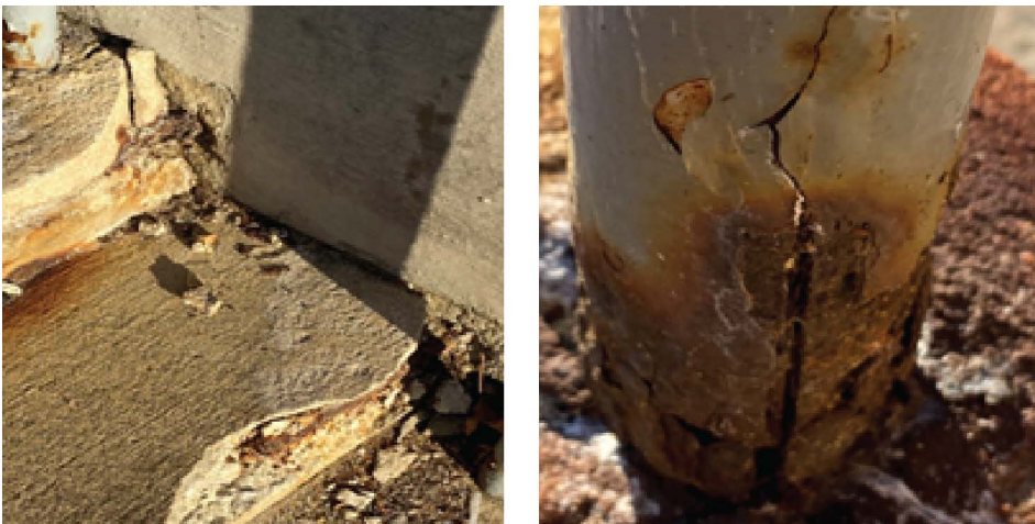
Figure 9. Crumbling Concrete and Rusted Railing
