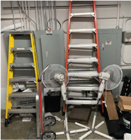
Figure 2. Blocked Electrical Panels
