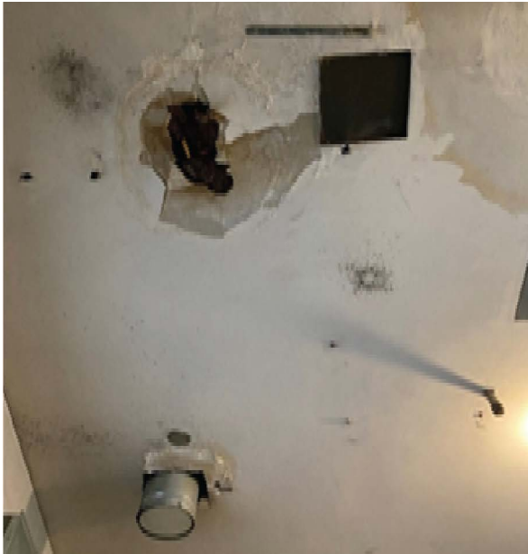
Figure 15. Holes in the Boiler Room Ceiling
