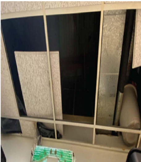
Figure 4. Missing Ceiling Tiles
