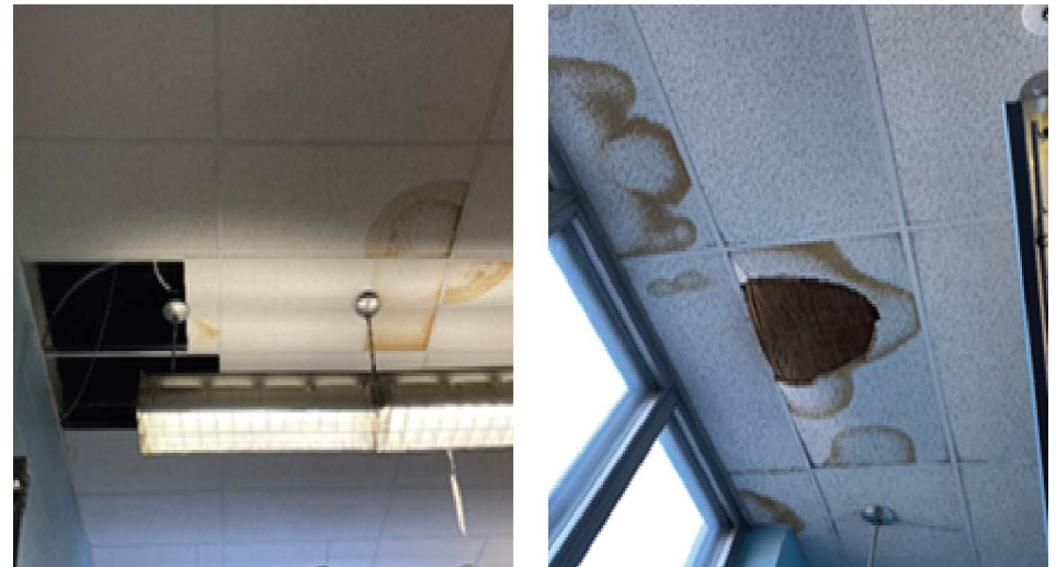
Figure 14. Issues with Ceiling Tiles in Workroom Area
