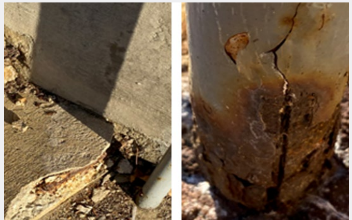
Figure 4. Crumbling Concrete and Rusted Railing
