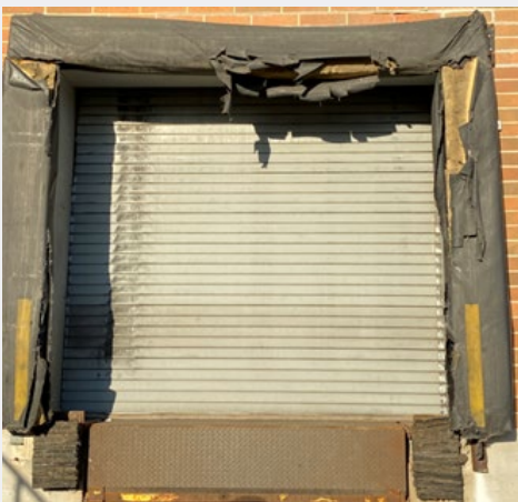
Figure 1. Padding Around Dock Door
