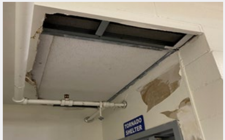
Figure 3. Gaping Hole in Ceiling
