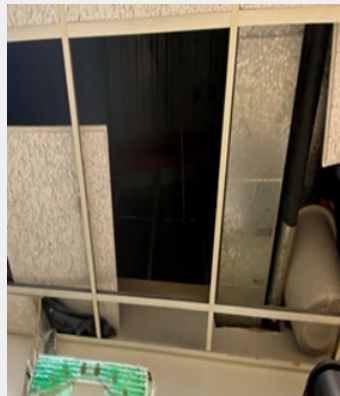
Missing Ceiling Tiles
