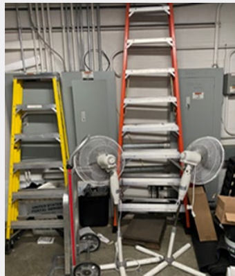
Blocked Electrical Panels
