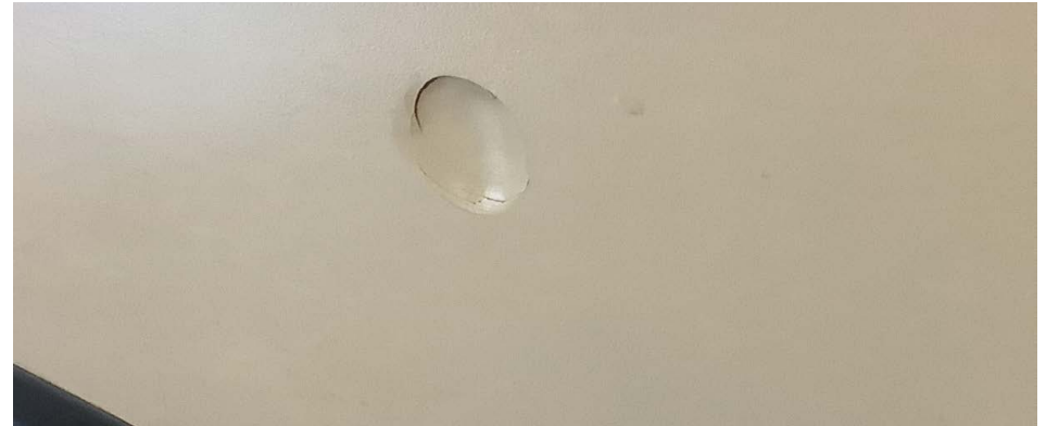
Hole in Wall Near PO Box Section of the Retail Lobby
