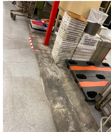
Missing Floor Tiles
