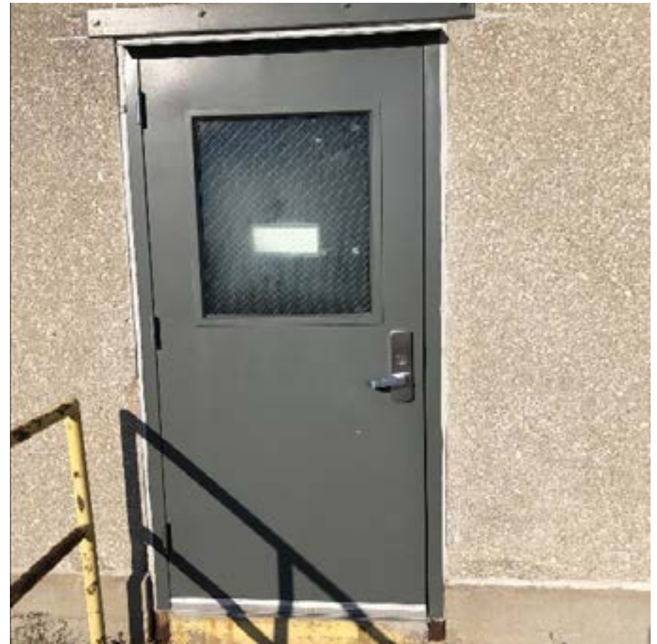
Figure 2. Exterior Door Without a Secure Access Badge Reader
