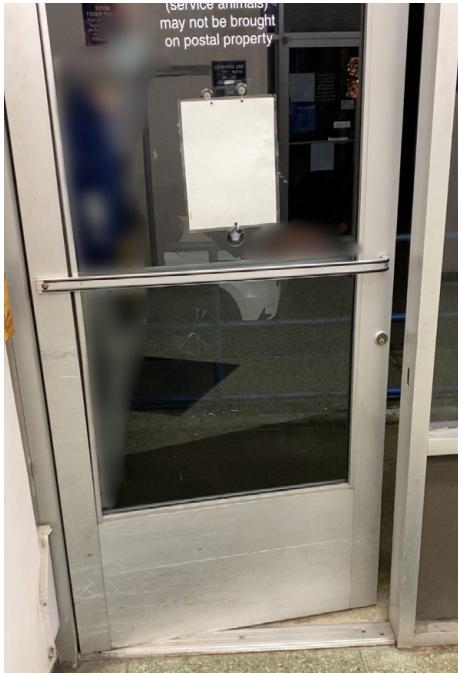
Source: OIG Photo taken November 30, 2021.
