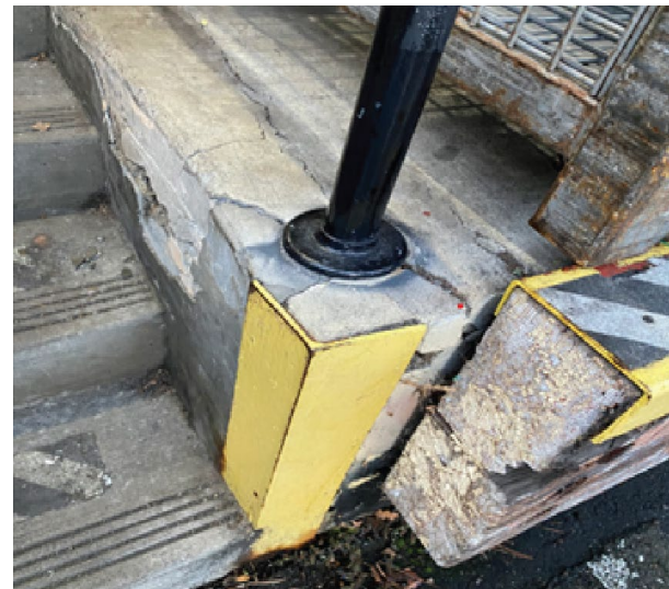
Figure 1. Crumbling Concrete on Dock
