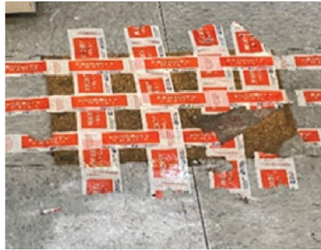
Figure 9. Damaged and Dirty Floors
