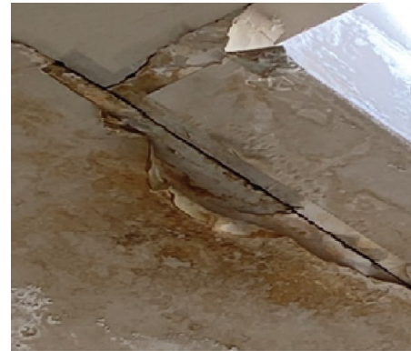
Figure 7. Stained and Peeling Ceilings
