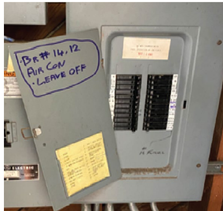
Figure 14. Broken Electrical Panel Door
