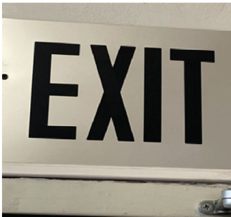
Figure 13. Exit Sign Not Illuminated
