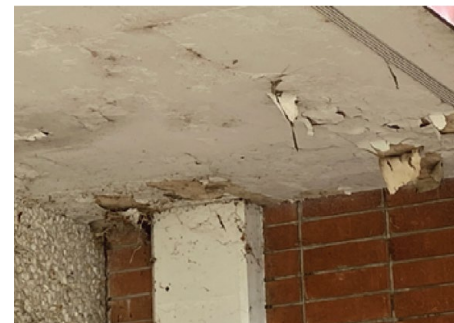
Figure 1. Peeling Paint and Holes
