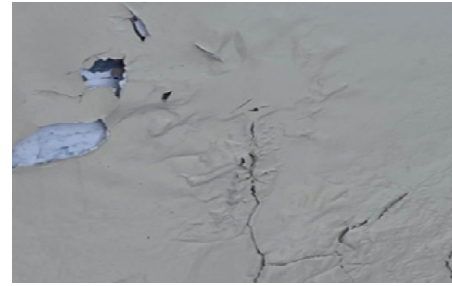
Figure 5. Peeling Paint and Holes in Walls
