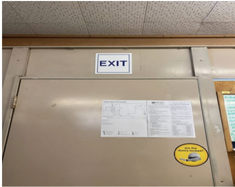
Figure 13. Non-Illuminated Exit Sign
