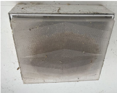
Figure 9. Dirty Lightbulb in Lobby Entrance
