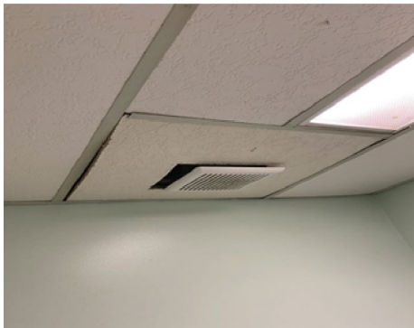
Figure 3. Misaligned Ceiling Vent in Restroom
