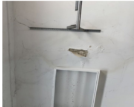
Figure 8. Damaged Ceiling in Loading Dock Area
