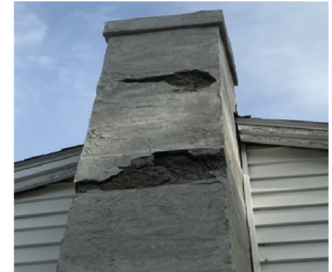
Figure 6. Damaged Chimney Wall
