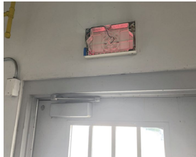
Figure 16. Missing Exit Sign Cover
