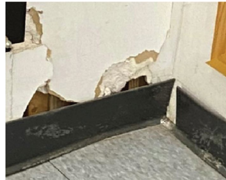
Figure 11. Damaged Wall in PO Box Area
