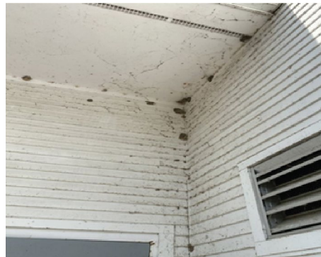
Figure 10. Cobwebs Around Main Entrance
