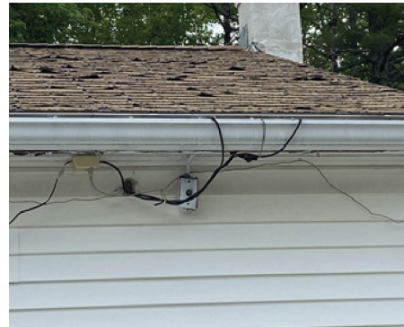
Figure 5. Loose or Damaged Shingles
