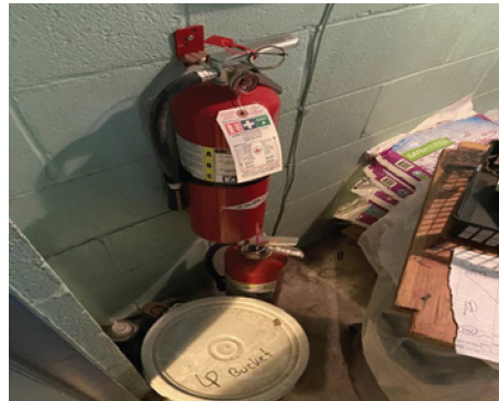
Figure 14. Blocked Fire Extinguisher
