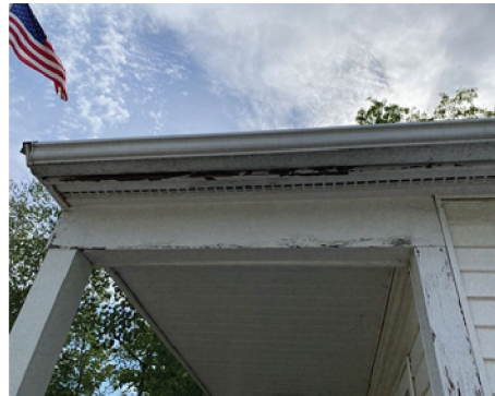
Figure 4. Exterior Walls Needing Repairs and Paint
