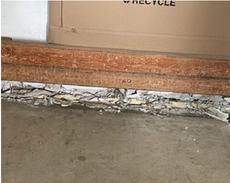
Figure 7. Damaged Wall in Loading Dock Area
