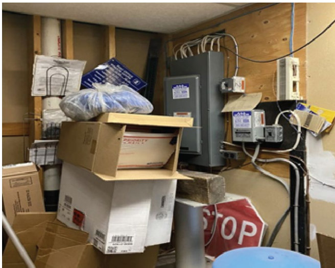
Figure 15. Blocked Electrical Panels
