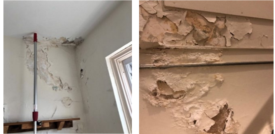
Figure 3. Walls with Holes and Peeling Paint and Plaster
