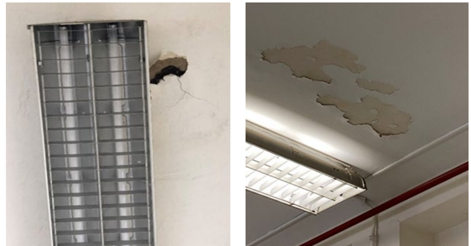
Figure 4. Ceilings with Holes and Peeling Paint and Plaster
