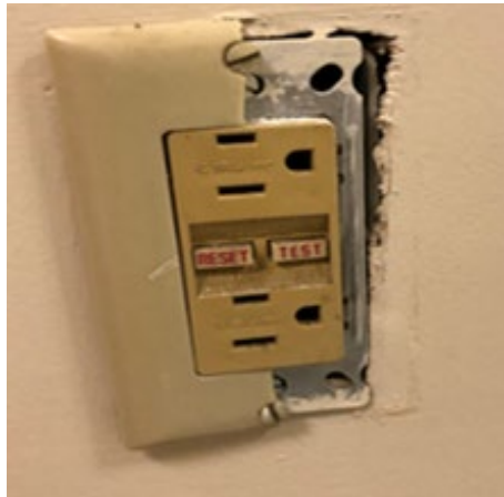
Figure 11. Broken Electrical Outlet in Restroom
