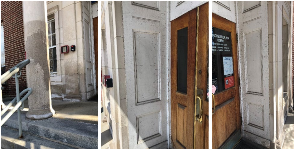
Figure 6. Front Entrance Columns, Archway, and Doors Need Painting
