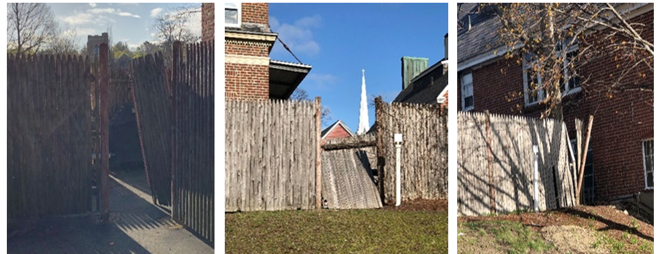
Figure 7. Damaged Wooden Fence
