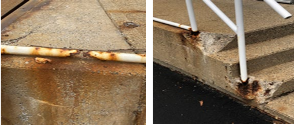
Figure 1. Rusted and Broken Railing with Steps Missing Cement
