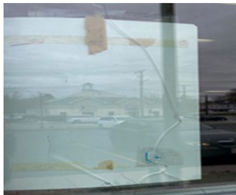
Figure 2. Broken Windowpane in Retail Lobby
