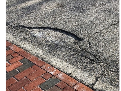
Figure 15. Pothole in Parking Lot
