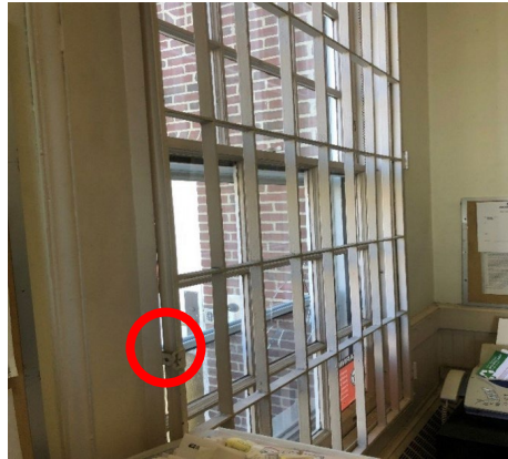
Figure 19. Missing Lock on Window Grate
