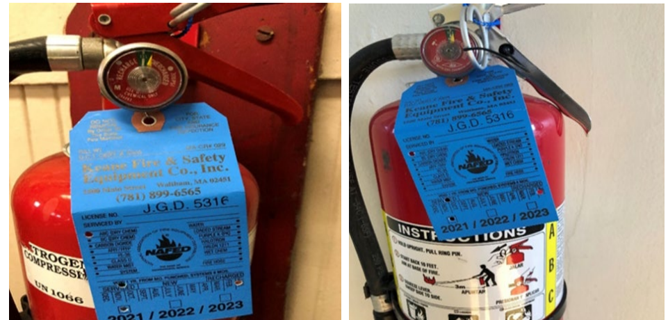
Figure 13. Fire Extinguishers with No Monthly Inspection Tags and Overcharged
