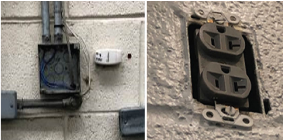
Figure 8. Exposed Electrical Box and Outlet
