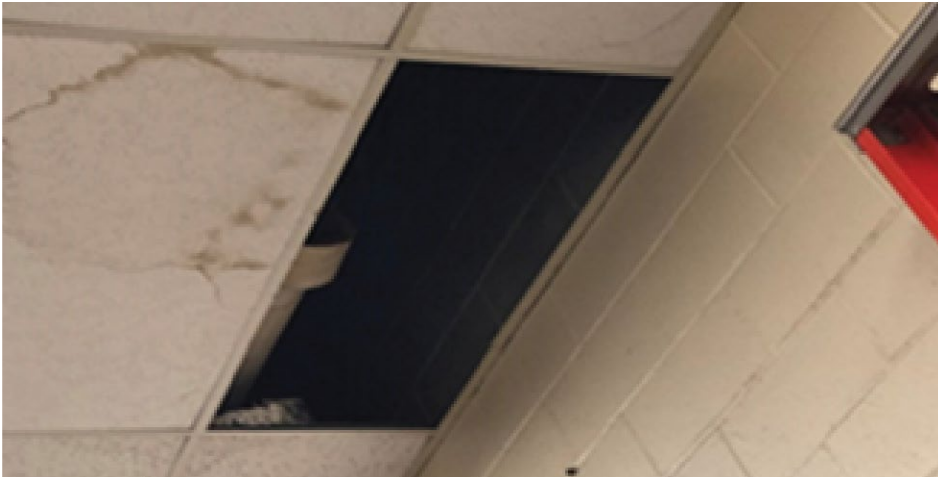
Figure 2. Missing and Stained Ceiling Tiles
