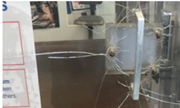
Figure 7. Cracked Retail Window
