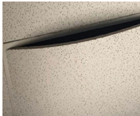
Figure 4. Misaligned Ceiling Tile
