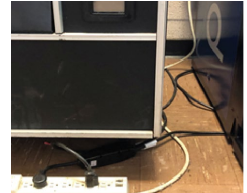
Figure 10. Vending Machines Plugged Into Surge Protector
