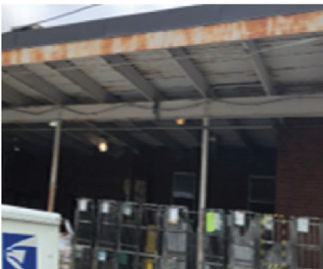
Figure 3. Rusted Exterior Trim
