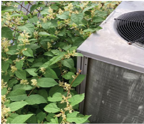
Overgrown vegetation near ventilation unit at Danvers Main Post Office, Danvers, MA. Photograph taken on September 21, 2021.
