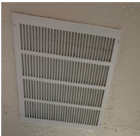
Return grille with no duct work at Wagram Main Post Office, Wagram, NC. Photograph taken on September 21, 2021.
