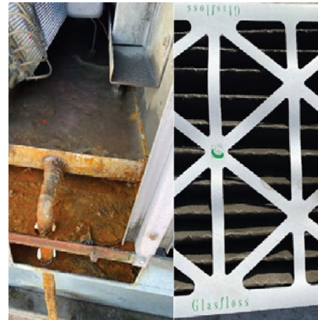
Clogged condensate pan and dirty filters at Stanton Main Post Office, Stanton, CA. Photograph taken on September 9, 2021.
