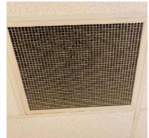
Dirty exhaust grille at Bettendorf Main Post Office, Bettendorf, IA. Photograph taken on September 13, 2021.
