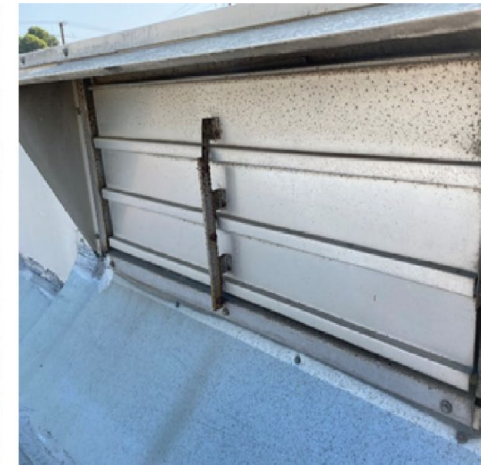
Closed outside air dampers at Mira Loma Main Post Office, Mira Loma, CA. Photograph taken on September 8, 2021.
