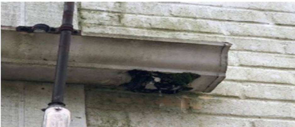
Figure 2. Missing Drain Spout
