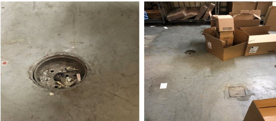
Figure 17. Uncovered Fixture on Floor
