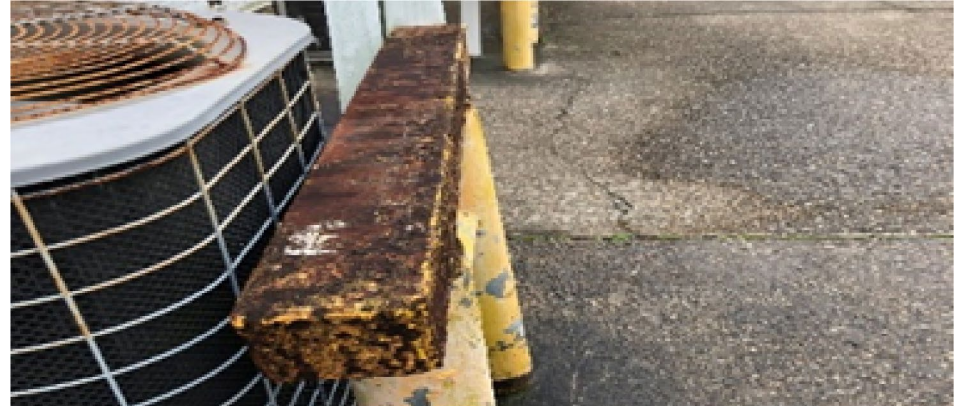
Figure 4. Rusted and Leaning Guard Rail for AC Unit
