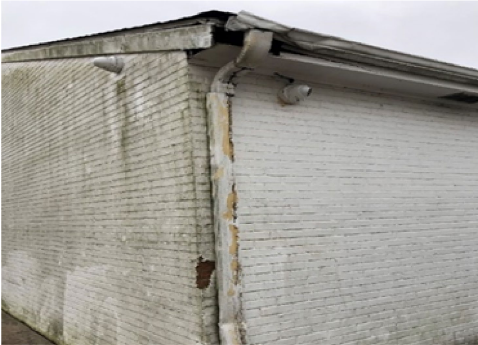
Figure 1. Rotted Wood and Damaged Gutter
