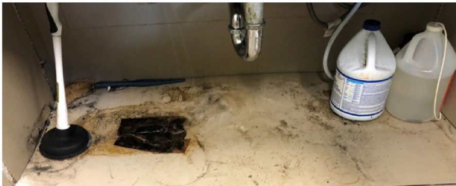
Figure 5. Potential Mold and Water Under Lunchroom Sink
