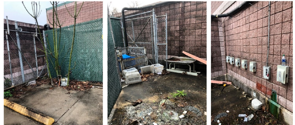
Figure 6. Tree Encroaching on Gas Meter and Excess Equipment and Trash in Fenced Area
