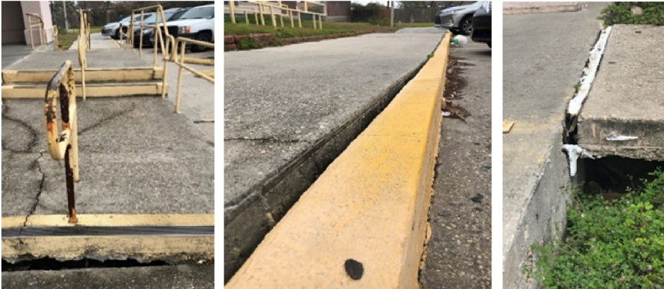
Figure 16. Cracked and Separated Entryway and Curb
