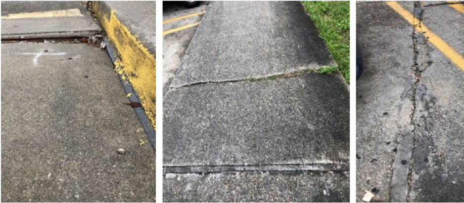
Figure 19. Walkway and Parking Lots with Cracks and Uneven Cement
