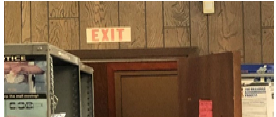
Figure 15. Exit Sign Not Illuminated
