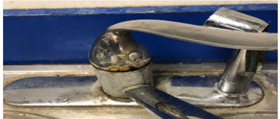
Figure 12. Dirty Sink and Fixture
