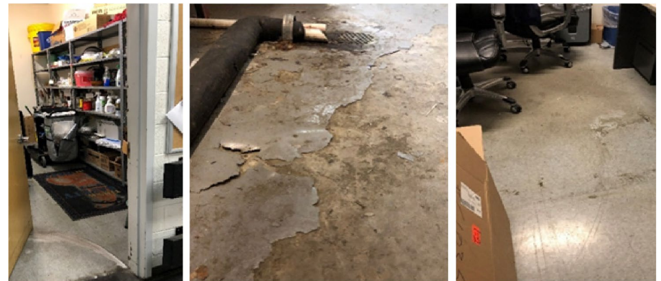
Figure 9. Scraped, Chipped, and Dirty Floors
