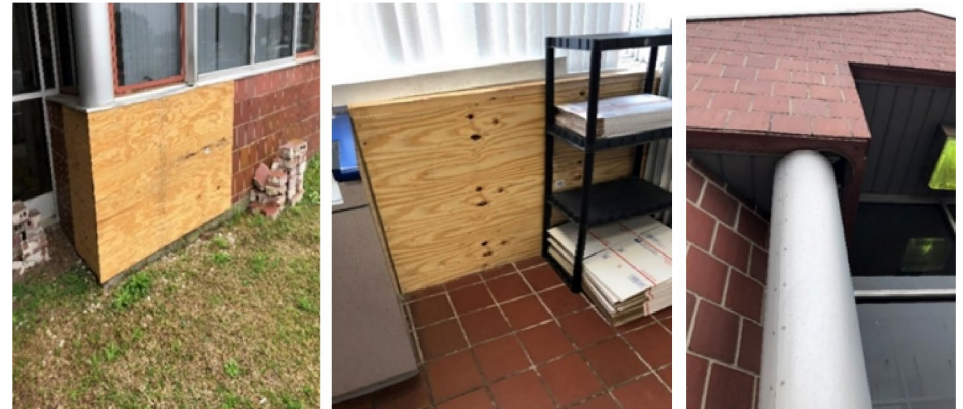
Figure 8. Damage to Building Structure
