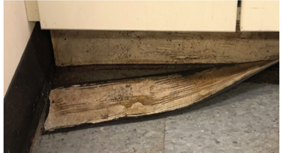
Figure 3. Partially Detached Baseboard Strip in Workroom
