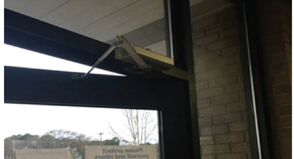
Figure 9. Damaged Door Closer at Lobby Entrance
