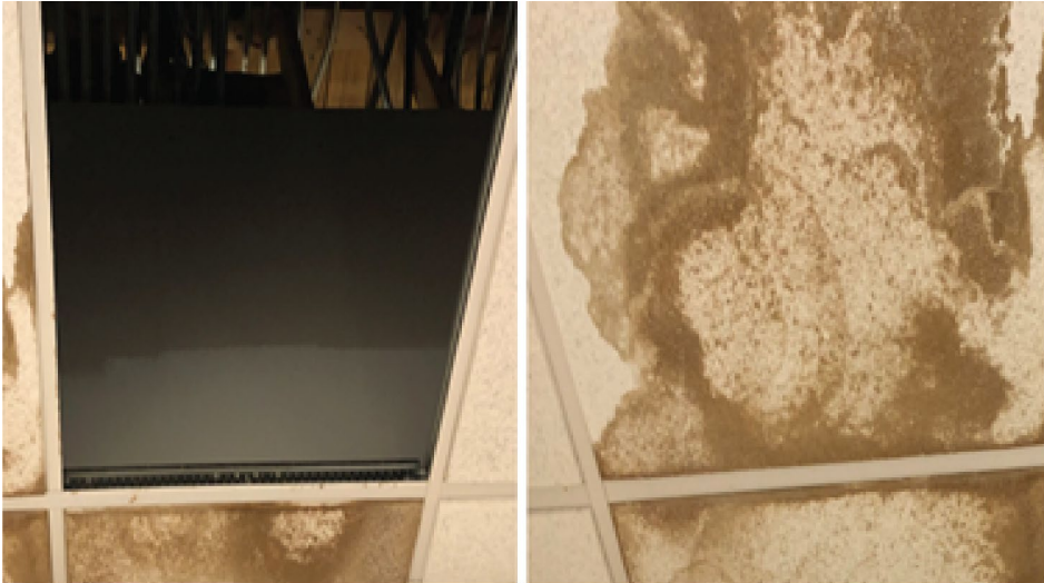
Figure 1. Missing and Stained Ceiling Tiles in Men's Restroom
