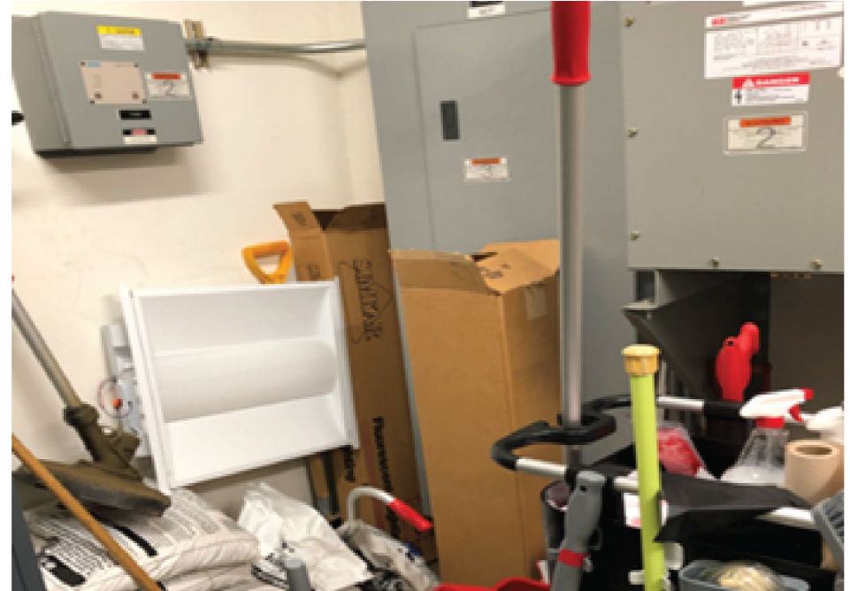
Figure 14. Blocked Electrical Panel
