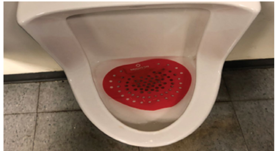
Figure 4. Semi-Operable Urinal in Men's Restroom
