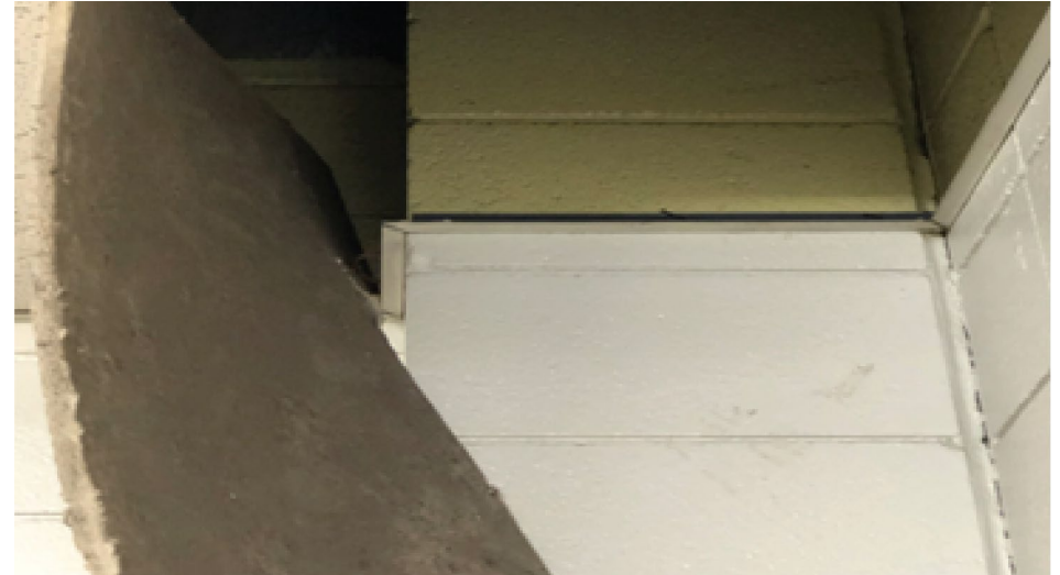
Figure 5. Hanging Ceiling Tile in Loading Dock
