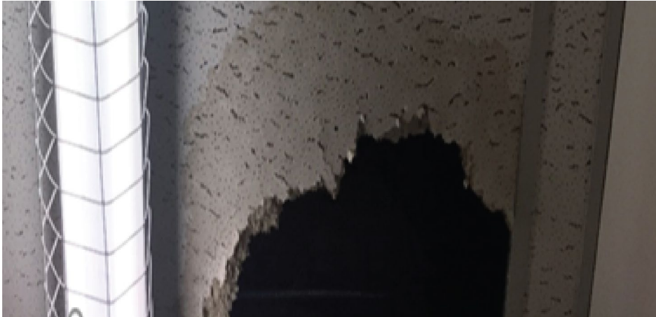
Figure 7. Damaged Ceiling Tile
