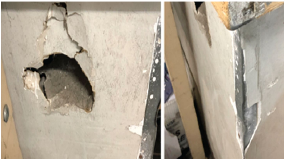
Figure 8. Damaged Walls in Workroom
