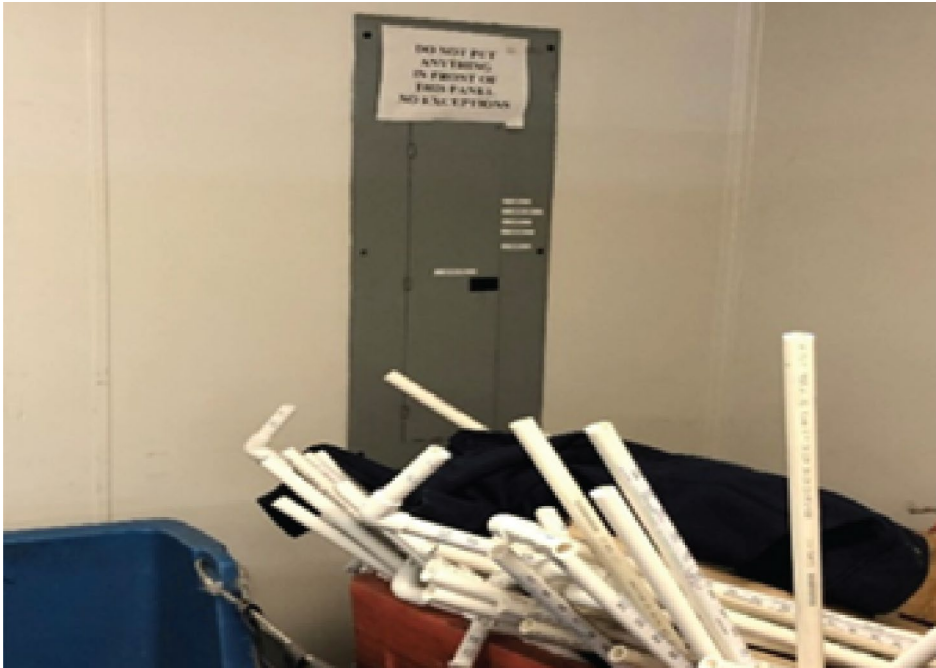
Figure 15. Blocked Electrical Panel
