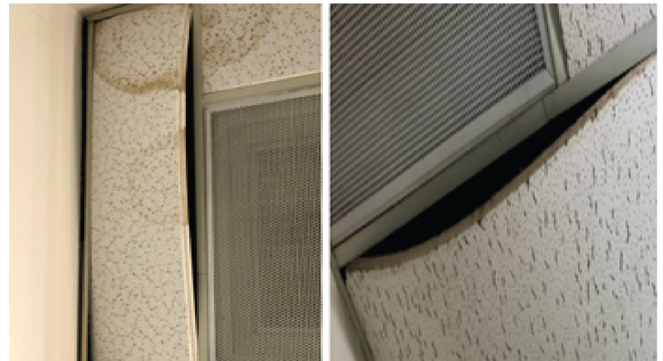
Figure 6. Bulging Ceiling Tiles
