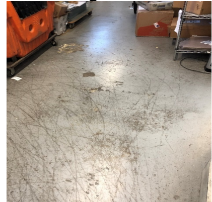
Figure 8. Dirty and Damaged Floors
