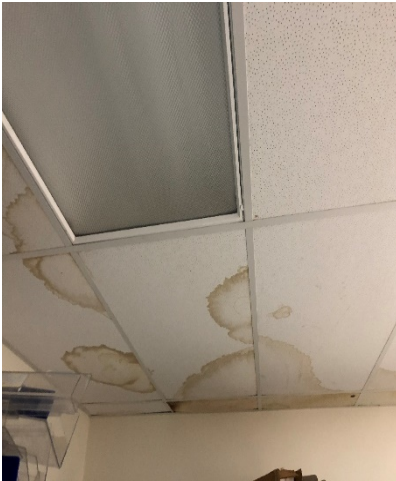
Figure 2. Stained Ceiling Tiles
