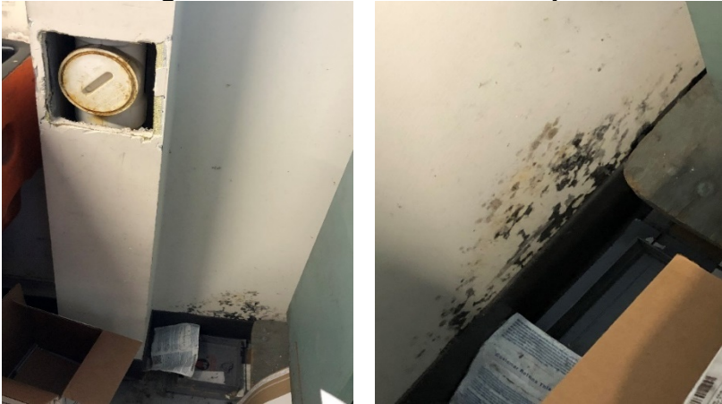
Figure 5. Potential Mold and Pipe
