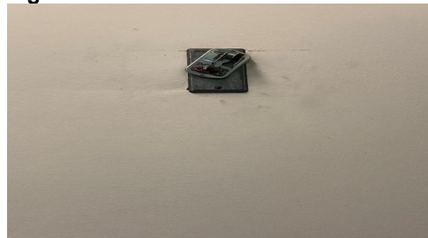
Figure 12. Uncovered Electrical Item
