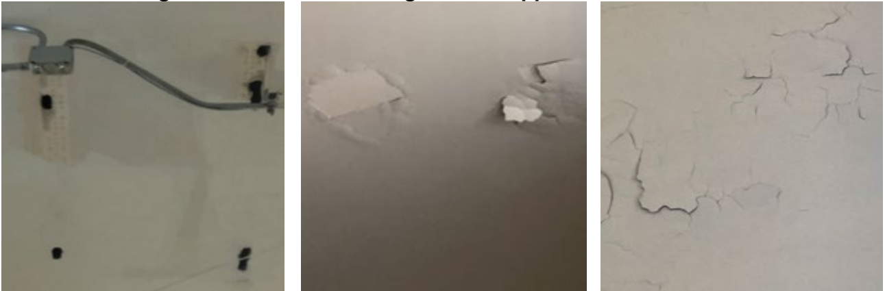
Figure 1. Walls and Ceilings with Chipped Paint and Holes
