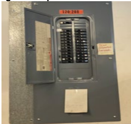
Figure 9. Open Electrical Panel
