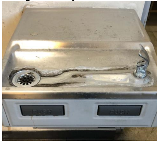
Figure 7. Dirty Water Fountain
