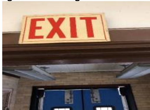
Figure 11. Exit Sign Not Illuminated
