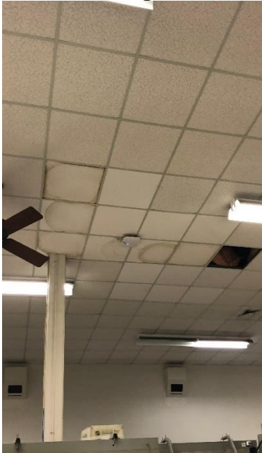
Figure 3. Stained/Missing Ceiling Tile
