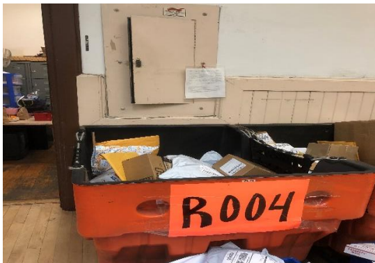
Figure 10. Open and Blocked Electrical Panel
