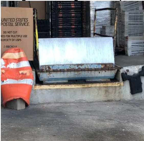
Figure 8. Missing Dock Bumper
