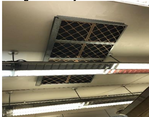
Figure 1. Dirty HVAC Filters
