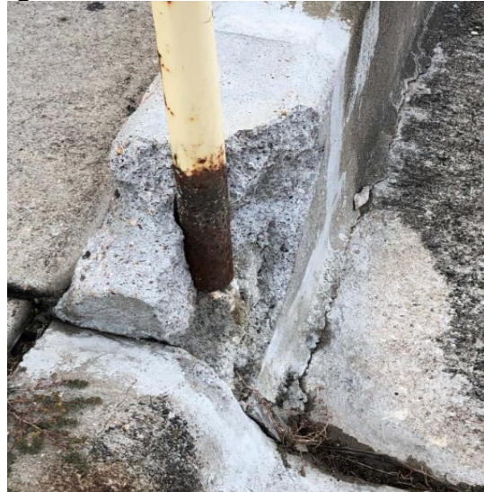
Figure 9. Broken Concrete Near Railing
