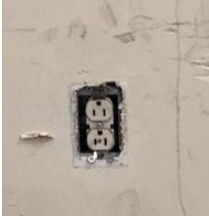
Figure 16. Missing Electrical Outlet Cover
