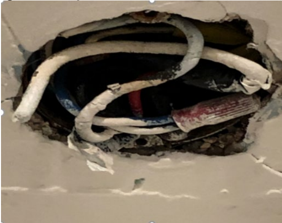
Figure 10. Exposed Wires in Ladies' Restroom
