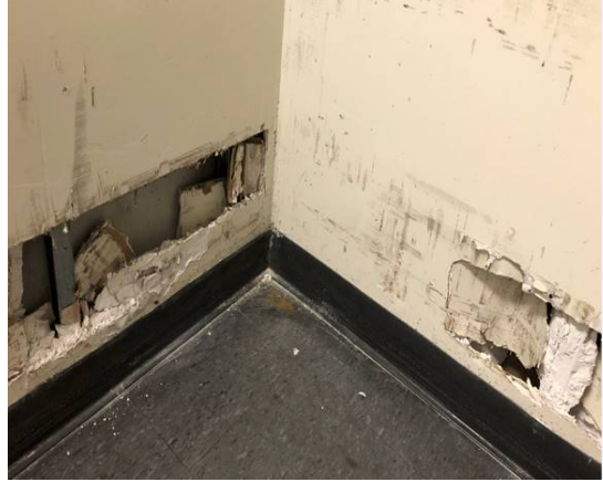
Figure 9. Damaged Walls Near Vault
