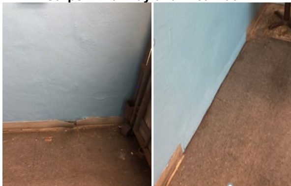
Figure 1. Damaged and Missing Baseboard Strips in Hallway and Breakroom
