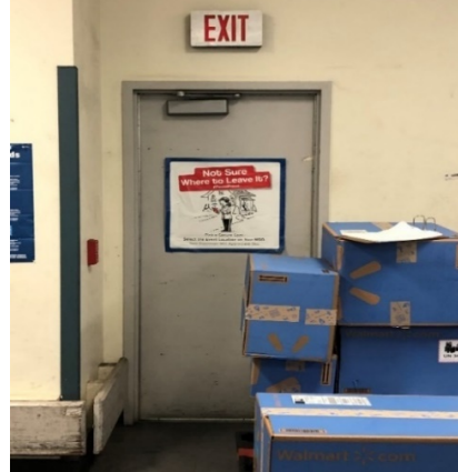
Figure 17. Blocked Exit Door
