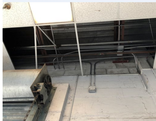
Figure 5. Missing Ceiling Tiles in Loading Dock Area
