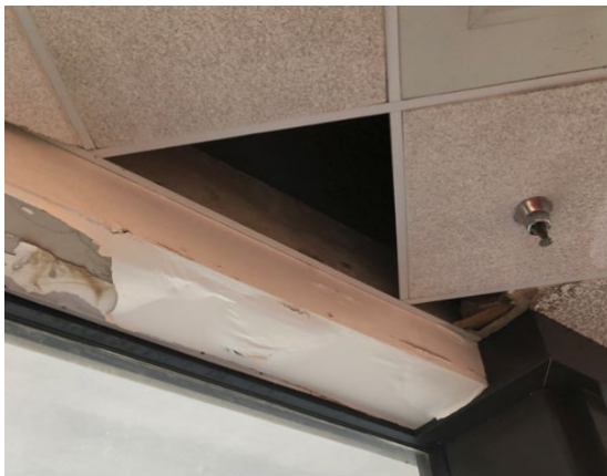
Figure 4. Missing Ceiling Tile in Post Office Box Area
