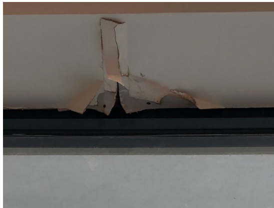
Figure 6. Damaged Wall in Customer Lobby
