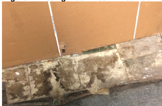
Figure 2. Missing Floor Tiles in Breakroom
