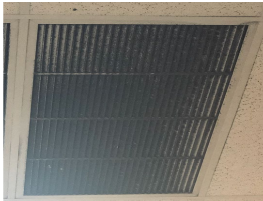
Figure 7. Dirty Air Vent in Customer Lobby
