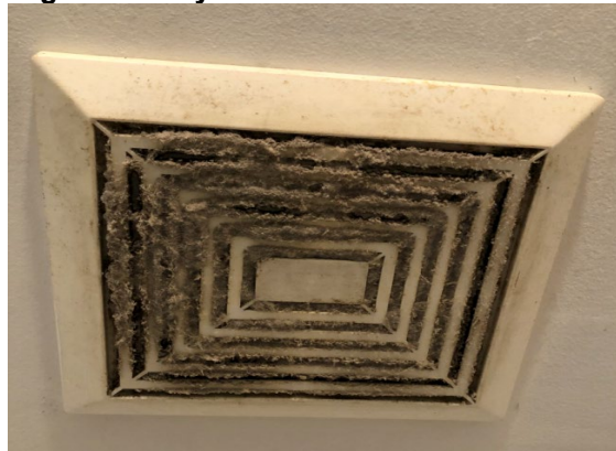
Figure 3. Dirty Air Vent in Ladies' Restroom
