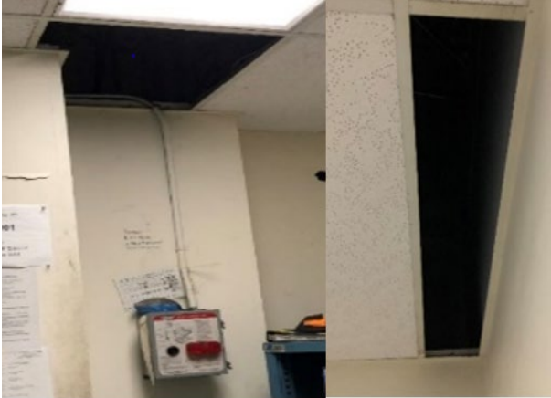
Figure 8. Missing Ceiling Tiles
