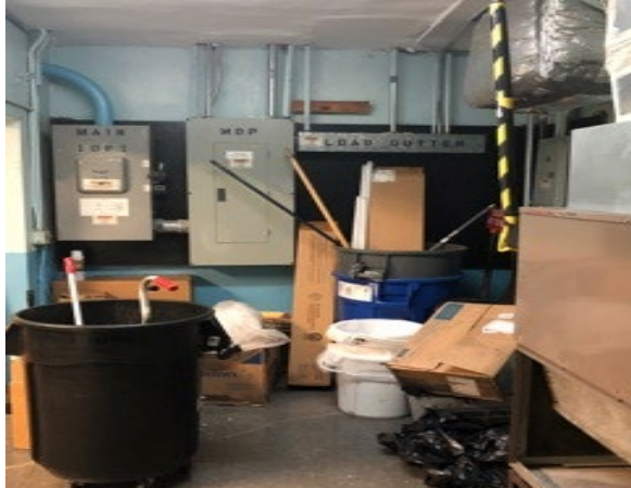
Figure 11. Blocked Electrical Panels
