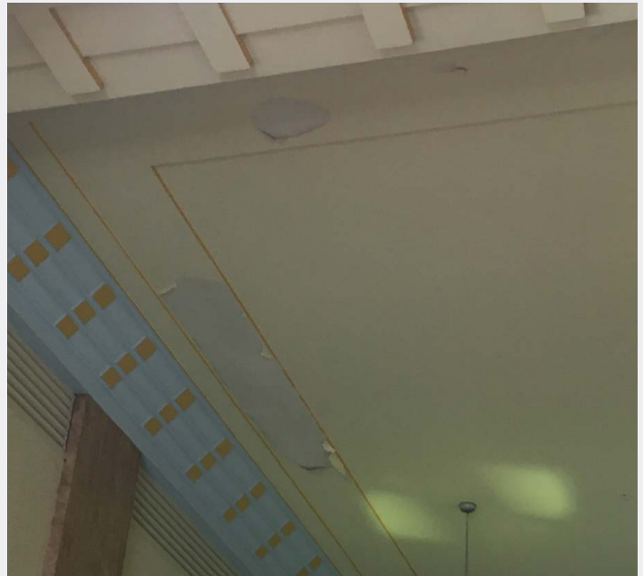
Figure 1. Peeling Paint in the Lobby and Workroom
