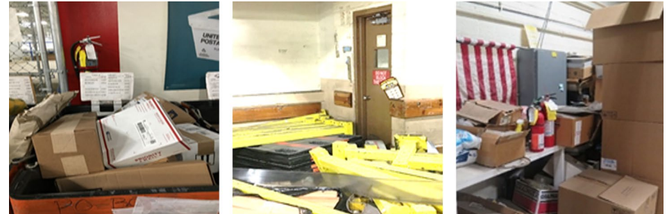
Blocked Fire Extinguisher
