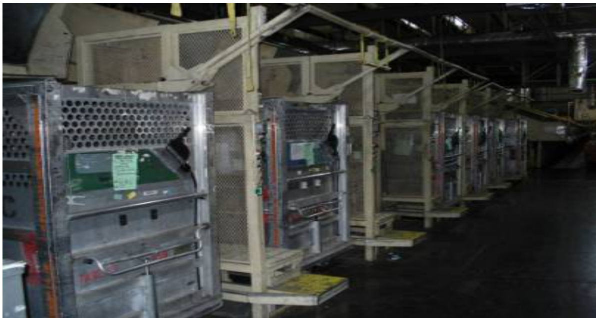
Illustration 7: Parcel Sorter Container Loaders were in poor working condition, resulting in many that could not be placed in a tilted position. The tilted position helps prevent damage to parcels as they are sorted into these containers from mail chutes.
