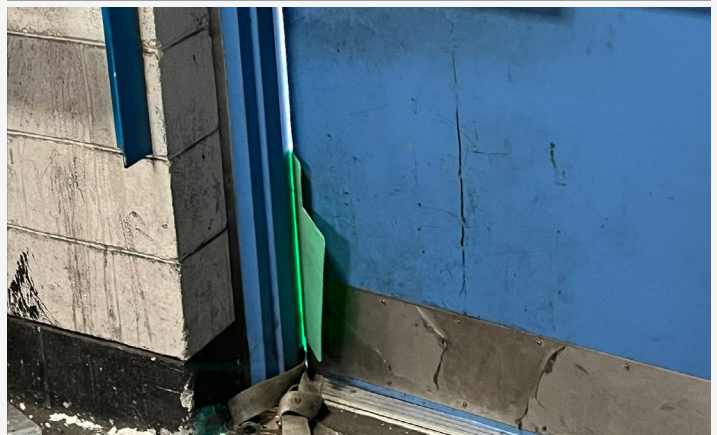
Figure 7. Door on the Dock Propped Open
