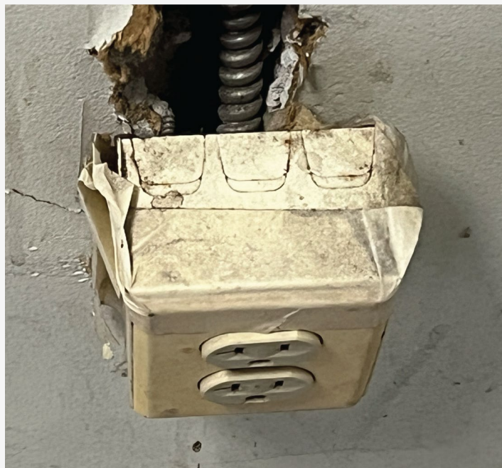
Figure 4: Dislodged Electrical Socket in Lobby
