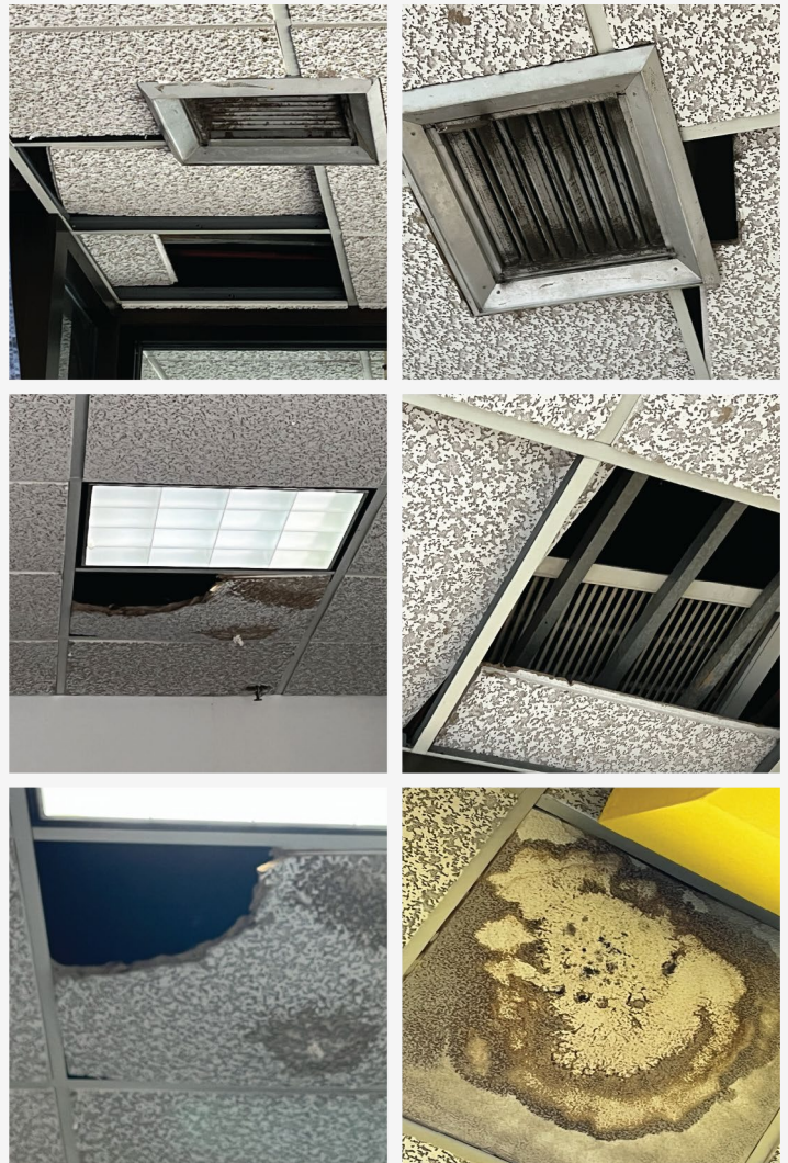
Figure 7: Missing, Broken, Misaligned, and Stained Tiles
