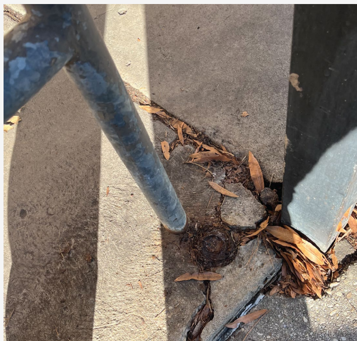
Figure 5: Broken Handrail in Dock Area
