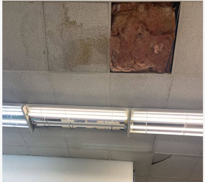
Figure 5. Example of Stained and Missing Tiles at the Lewiston MPO
