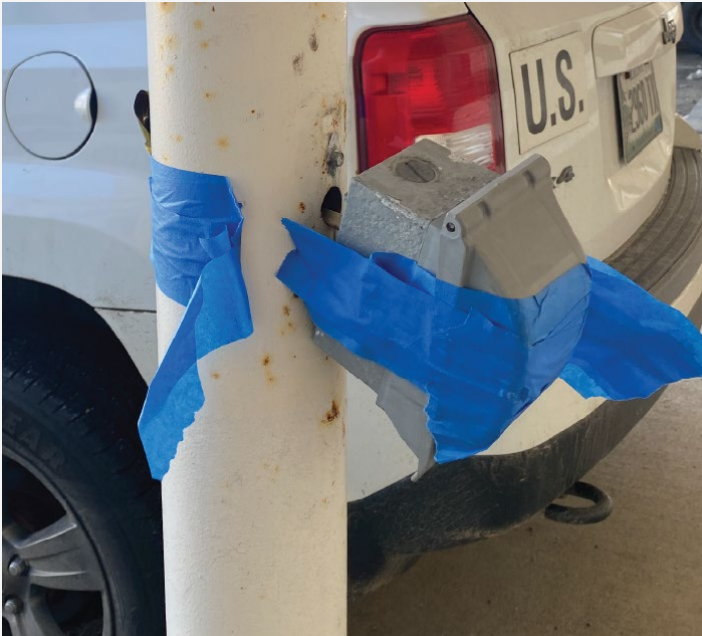
Figure 3. Broken and Unsecured Electrical Outlet at Industrial Park Annex
