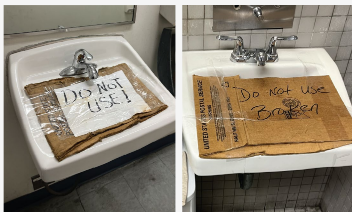
Figure 5. Inoperable Sinks in Men's and Women's Restrooms
