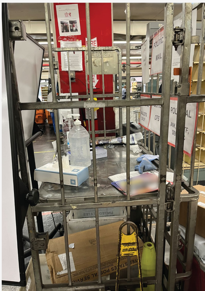
Figure 4. Blocked Fire Extinguisher in Workroom
