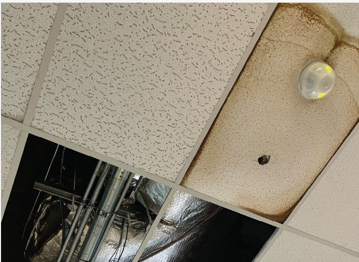
Figure 7. Missing Ceiling Tiles in Caller Services Office
