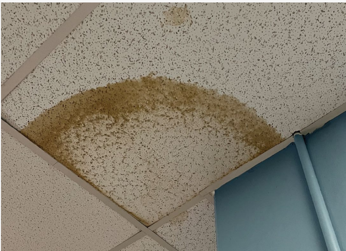
Figure 6. Stained Ceiling Tiles in Caller Services Office
